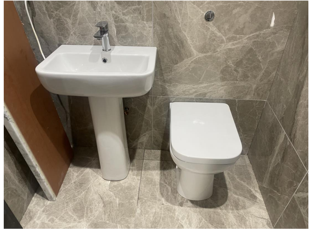
Ground Floor WC – Sanitary Items
