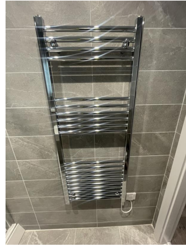
Residential Block – Towle radiator
