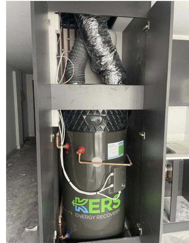
Residential Wing – KERS units installed
