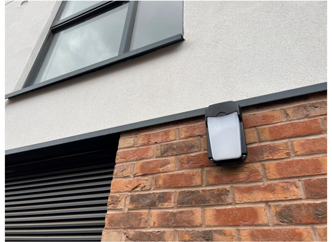
External light fittings
