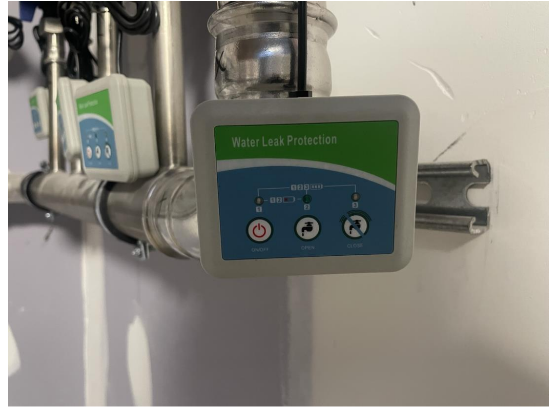
Residential Wing – Water leak protection
