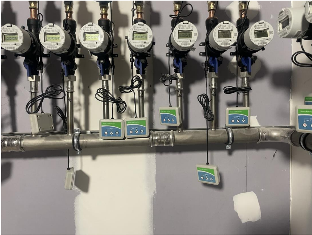
Residential Wing – Water leak protection
