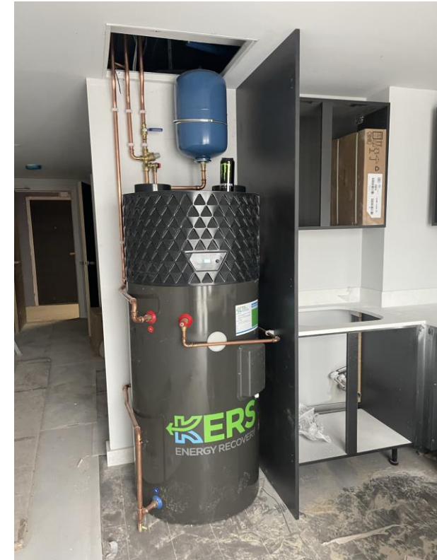
Residential Wing – KERS units installed
