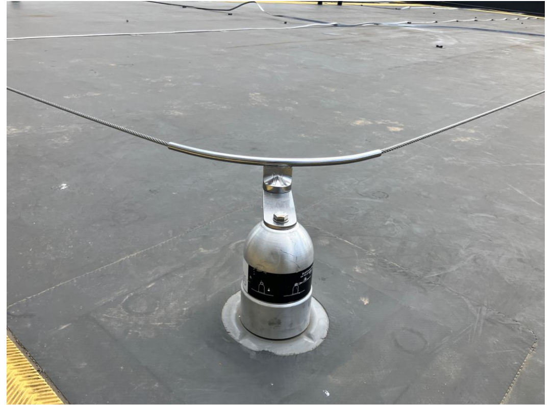
Student Wing – Mansafe system in place
