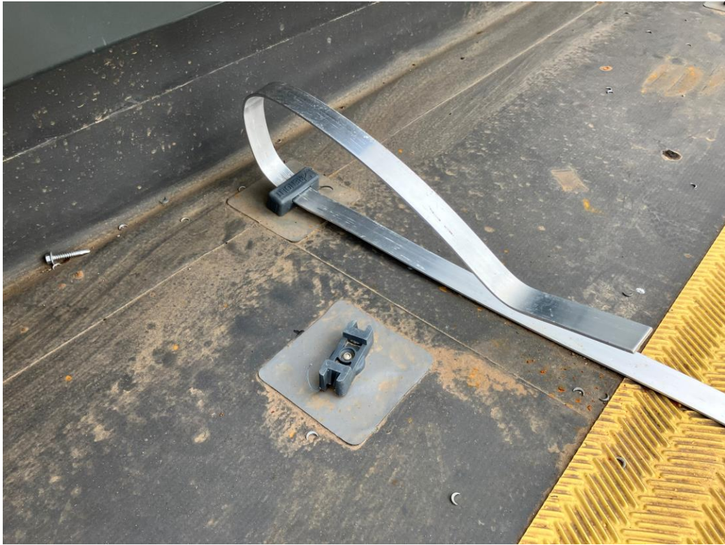
Residential Wing – Lightning protection cable
