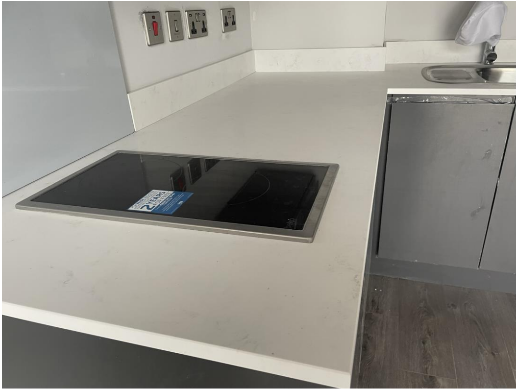
Residential Block – Appliances installed
