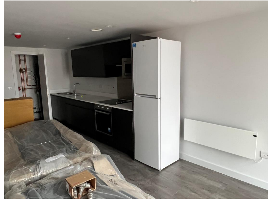
Residential Block – Fridge installed
