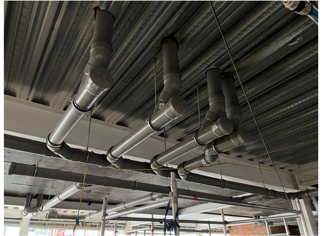
Residential Block – Above ground drainage
