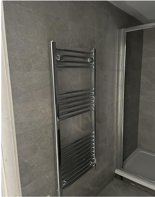
Residential Block – Towel radiator
