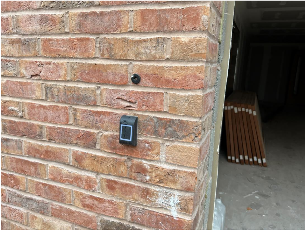
Residential Block – Fob access
