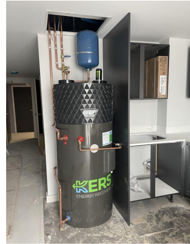
Residential Wing – KERS units installed
