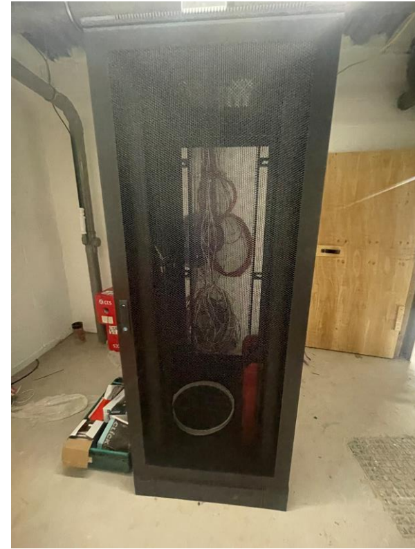
Residential Block – Data hub installed
