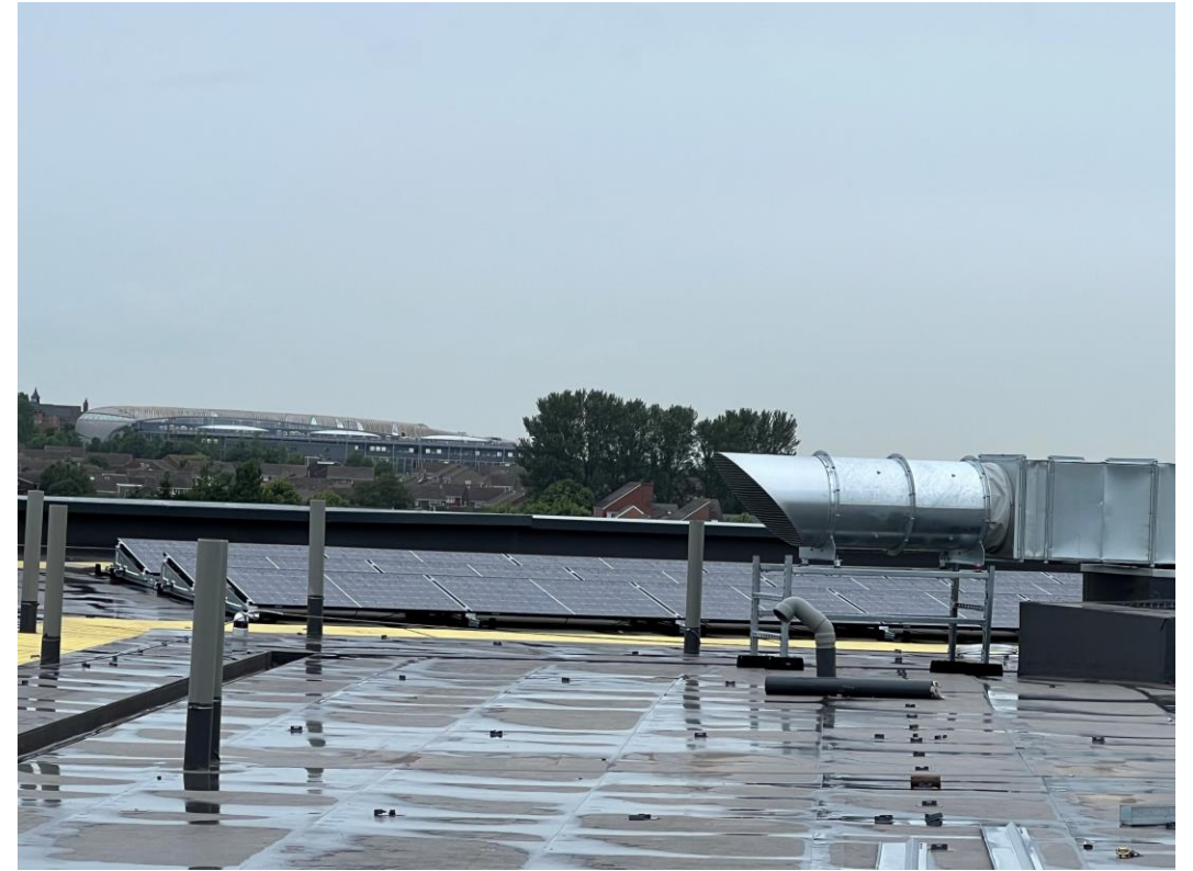
Student Wing – PV Panels
