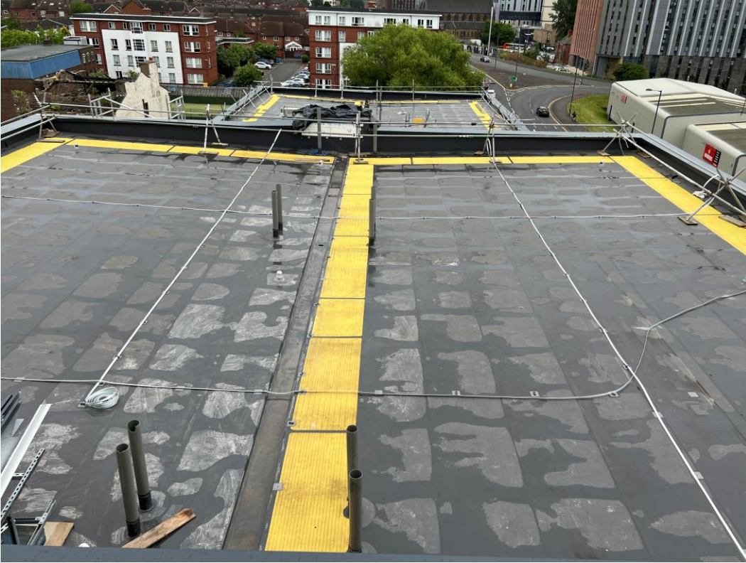
Residential Wing – Lightning protection cable
