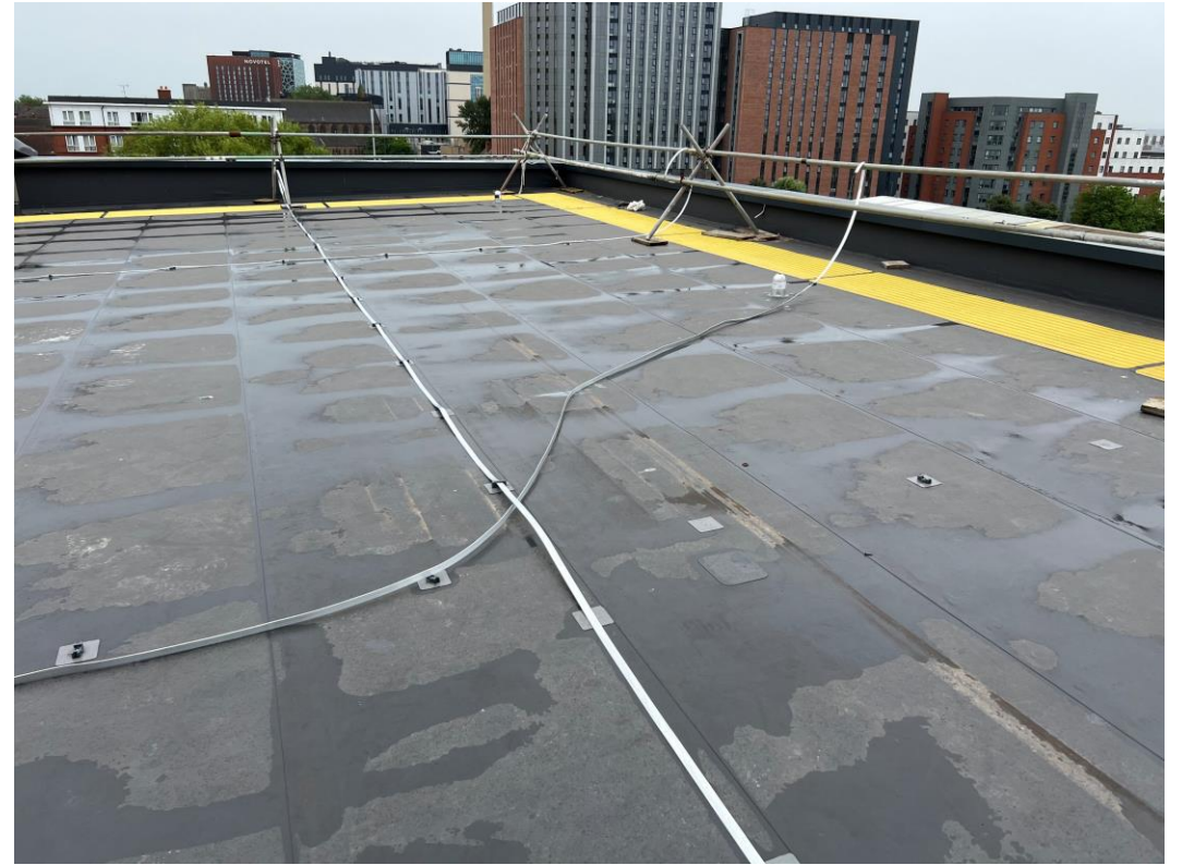
Residential Wing – Lightning protection cable
