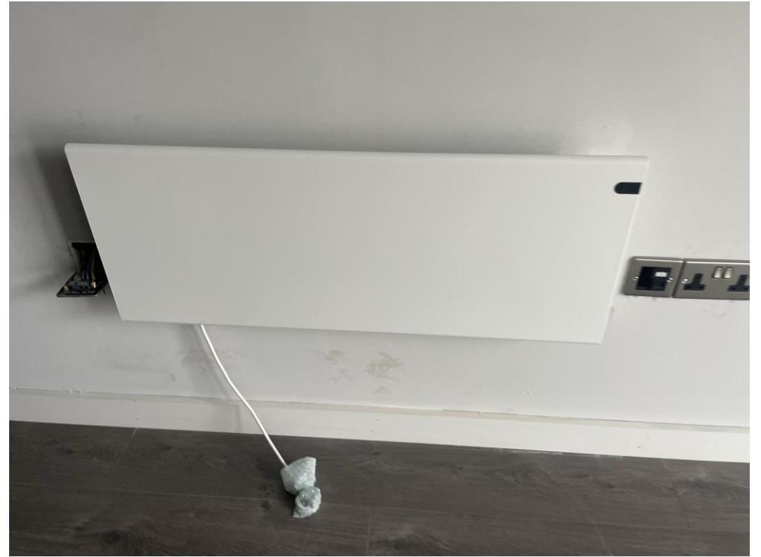
Residential Block – Panel heater
