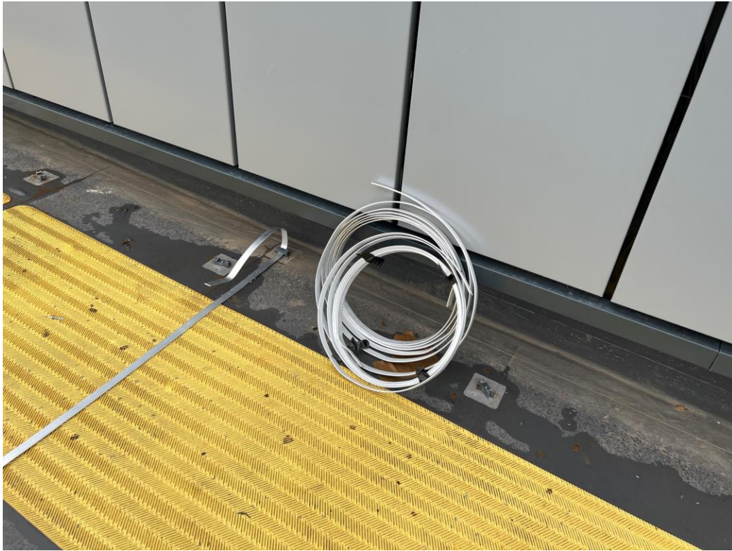
Residential Wing – Lightning protection cable
