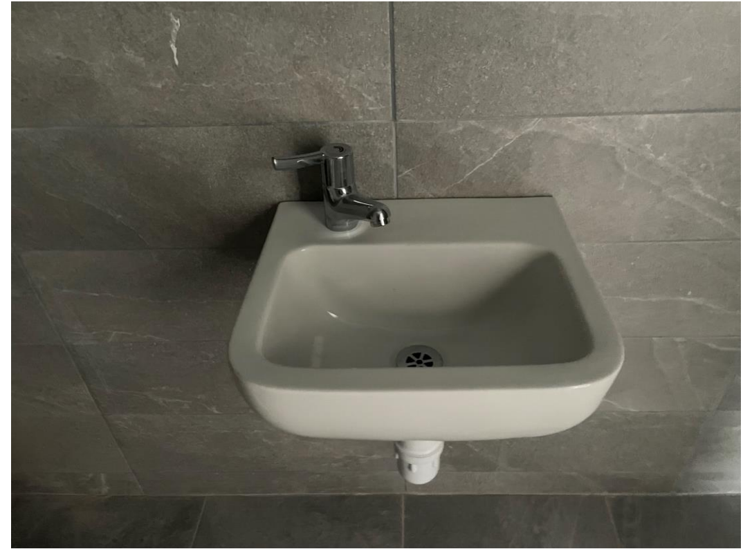
Residential Block – Sanitary appliances installed
