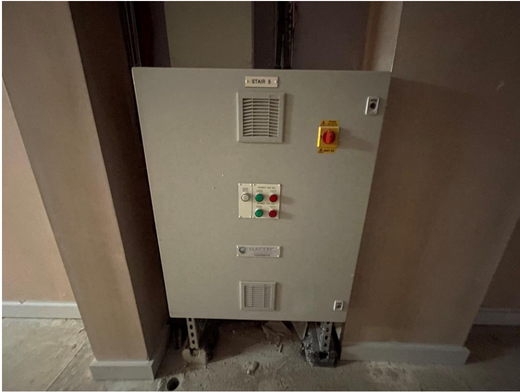
Residential Block – Smoke control system installed
