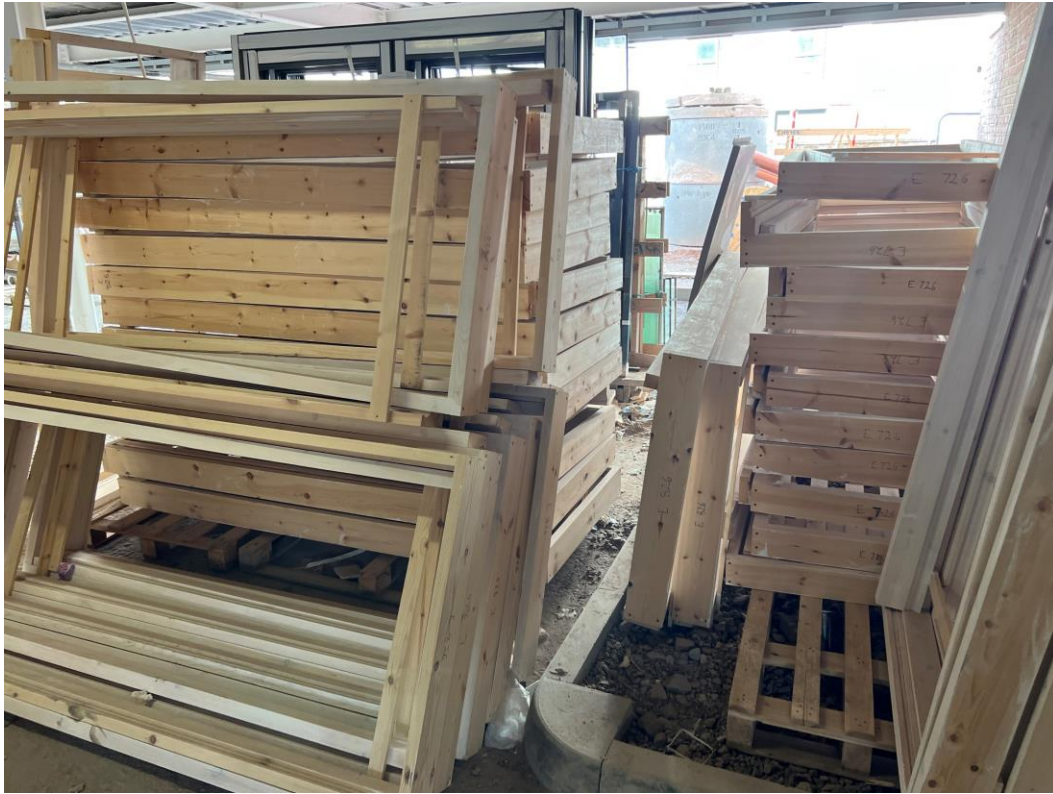
Material storage – Door Frames
