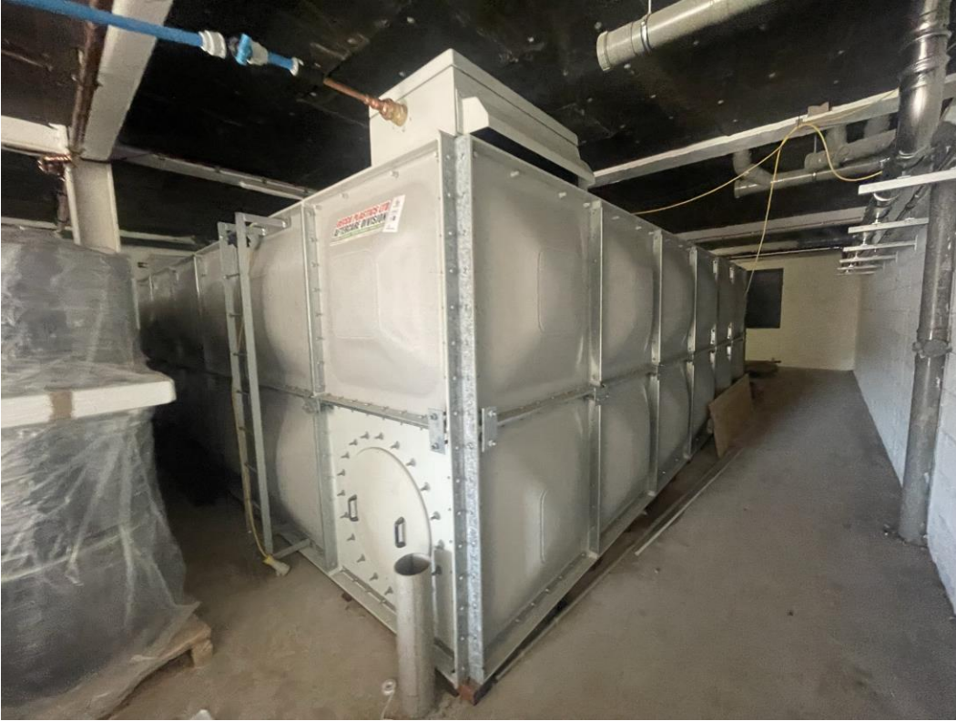
Residential Block – Water tank installed & filled
