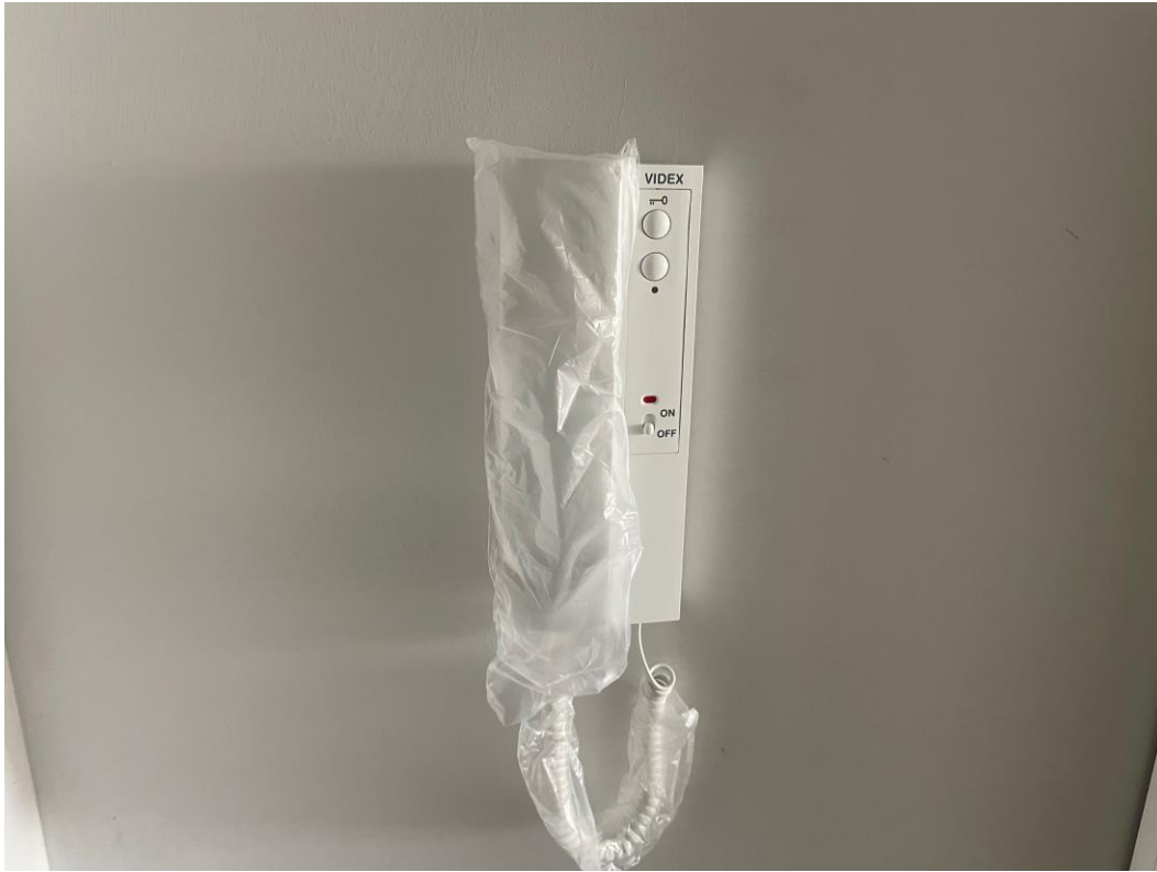
Residential Block – Intercom installed
