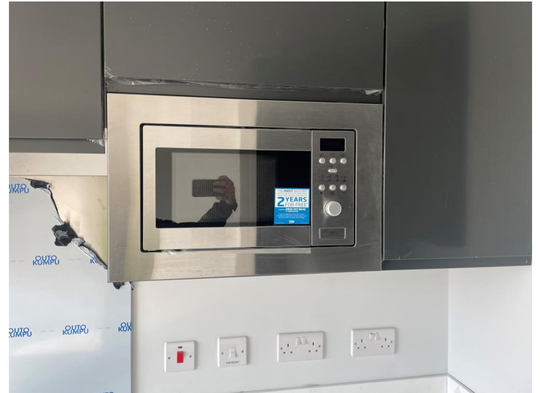
Residential Block - Microwave
