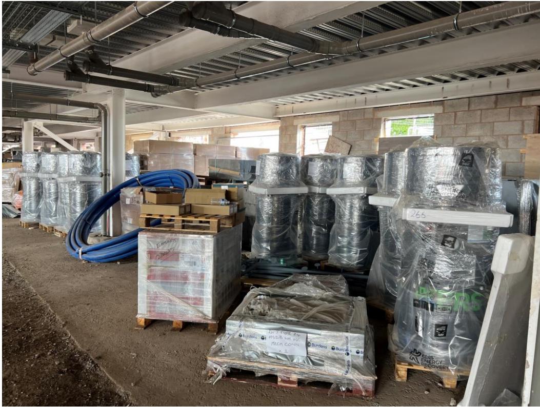
Materials Stored – KERS Units
