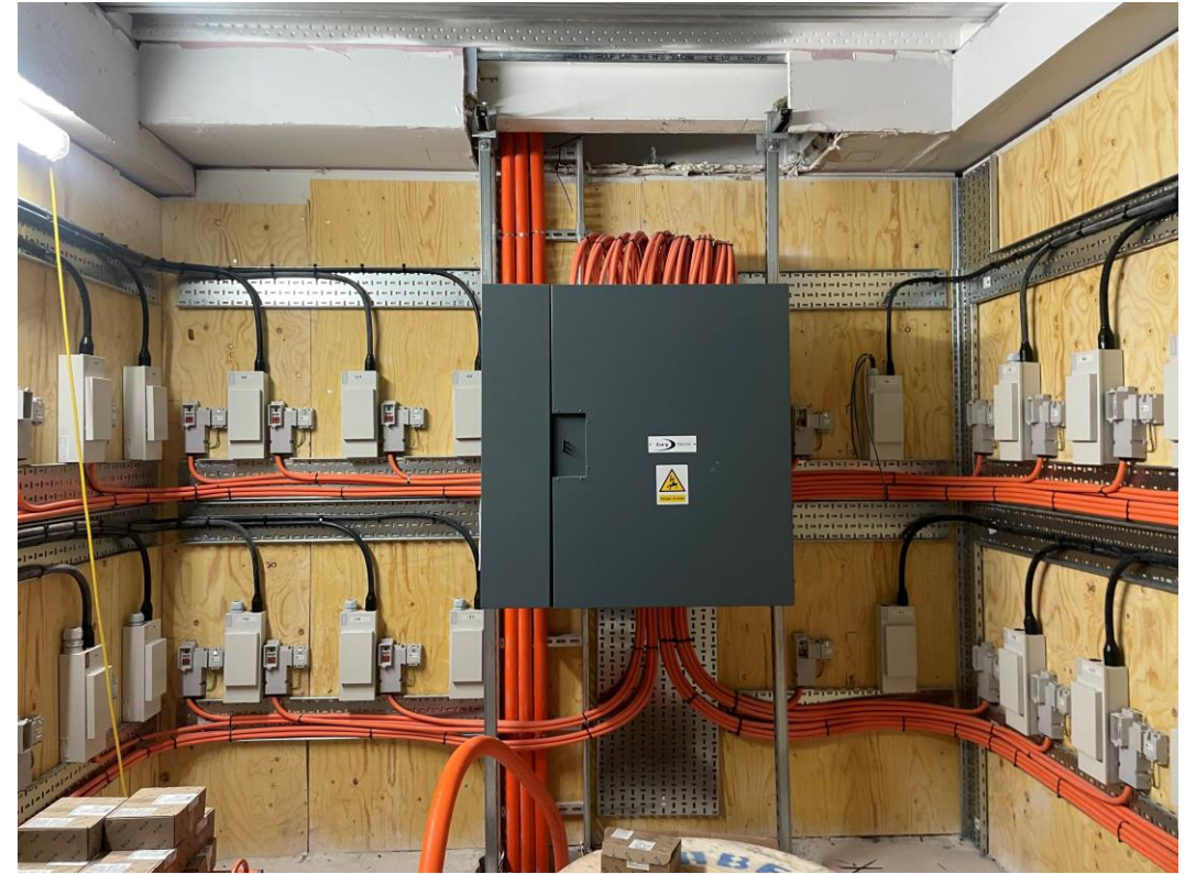
Residential Block – Apartment electrical meters
