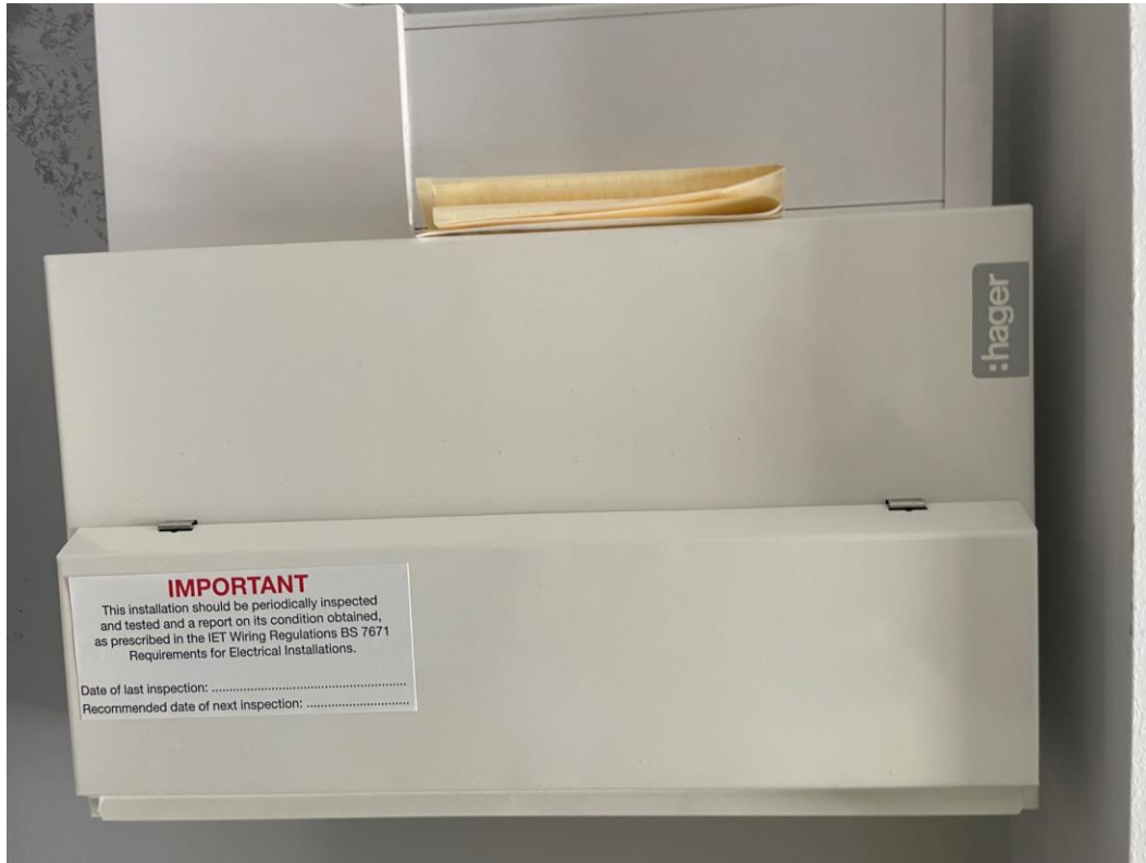
Residential Block – Electrical consumer unit
