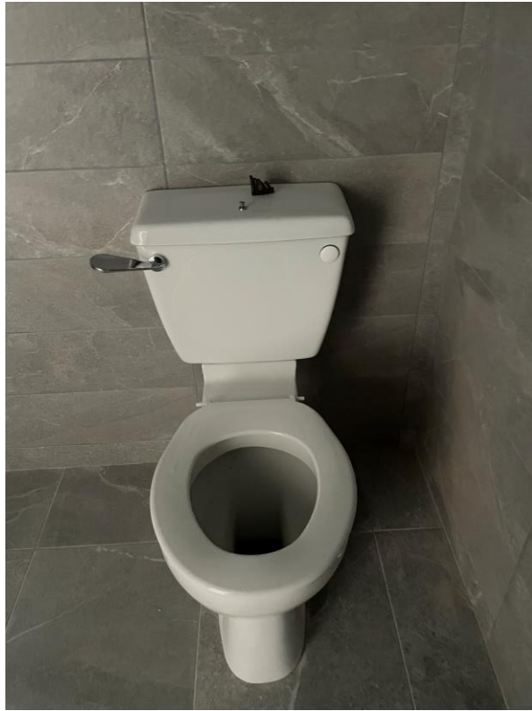
Residential Block – Sanitary appliances installed
