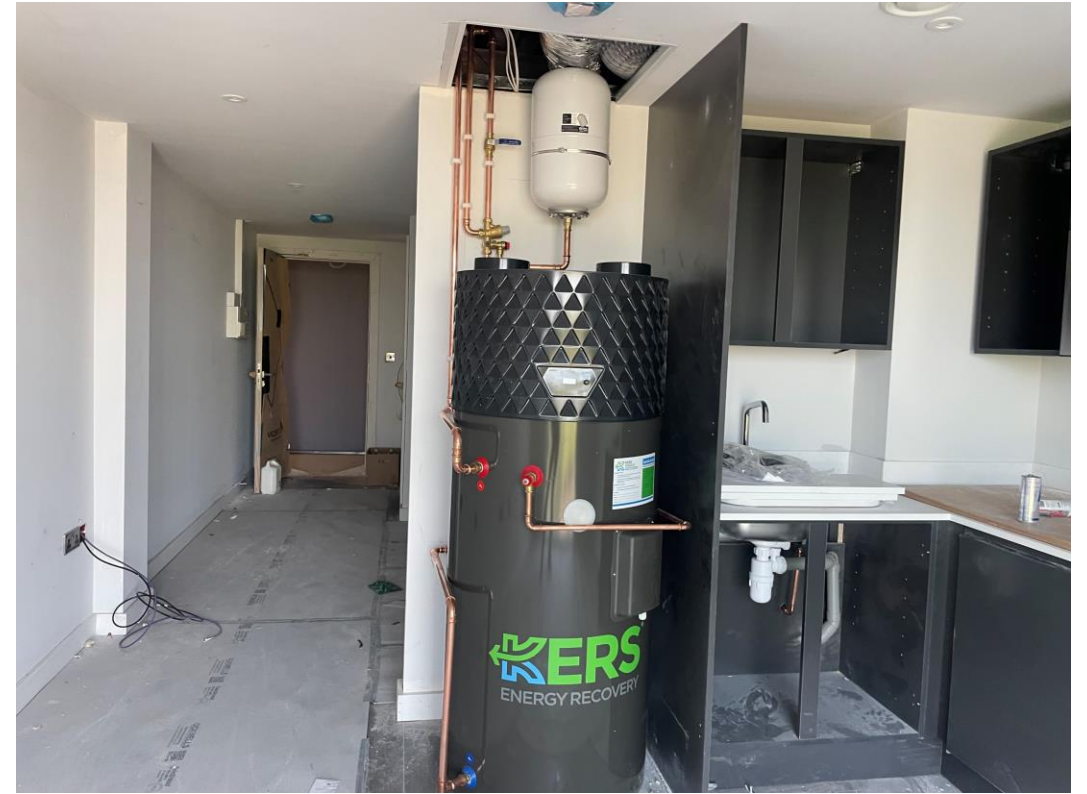
Residential Wing – KERS units installed
