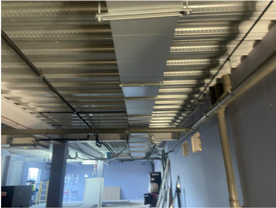
Residential Wing – Mechanical Ducting
