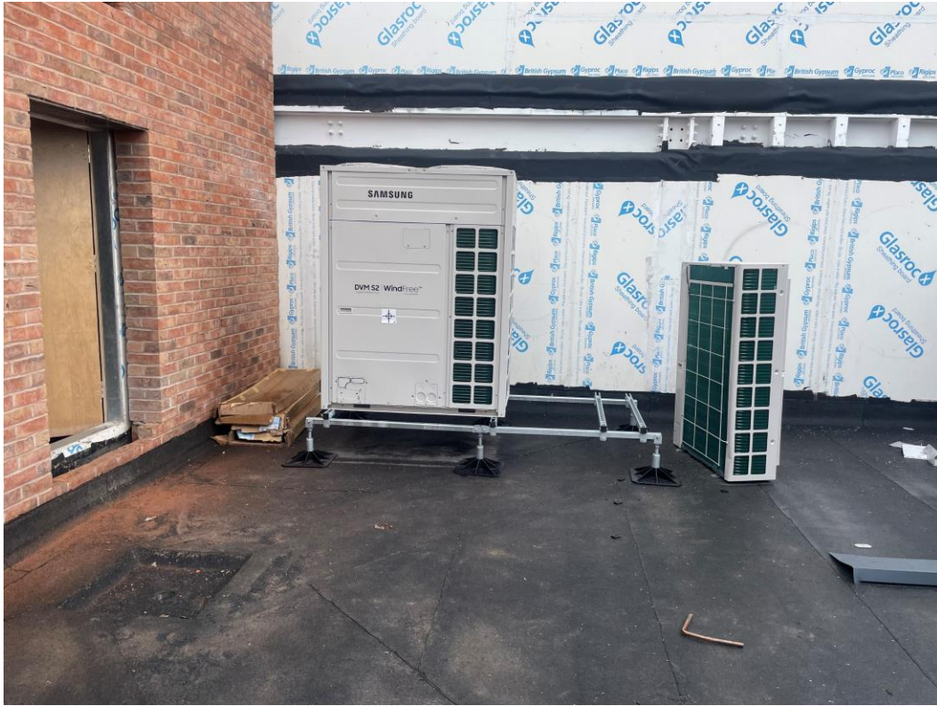
Residential Wing – Samsung air conditions units
