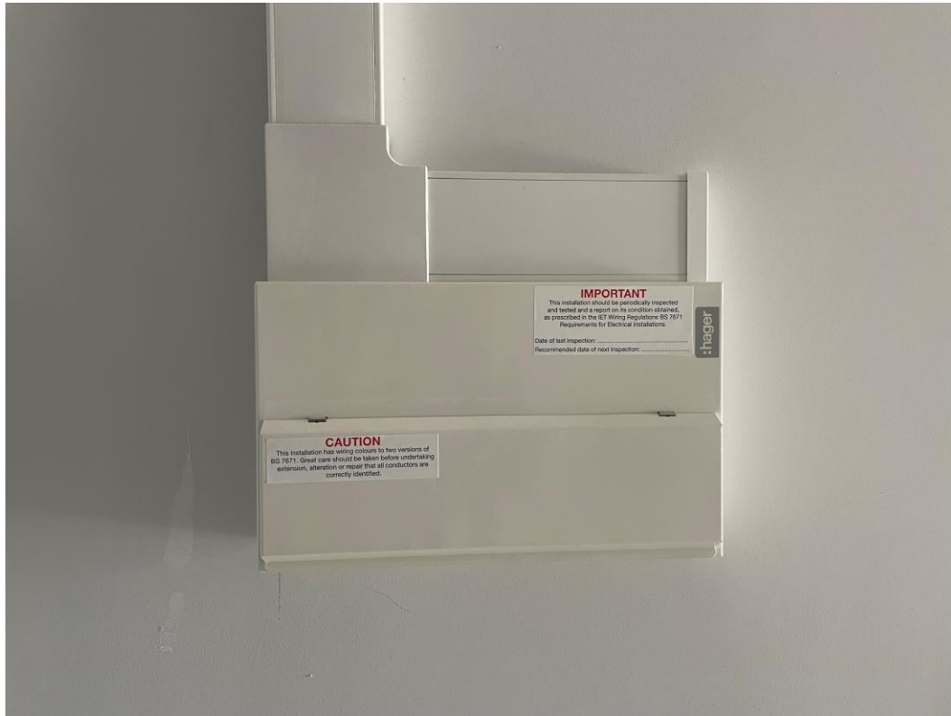
Residential Block – Electrical consumer unit
