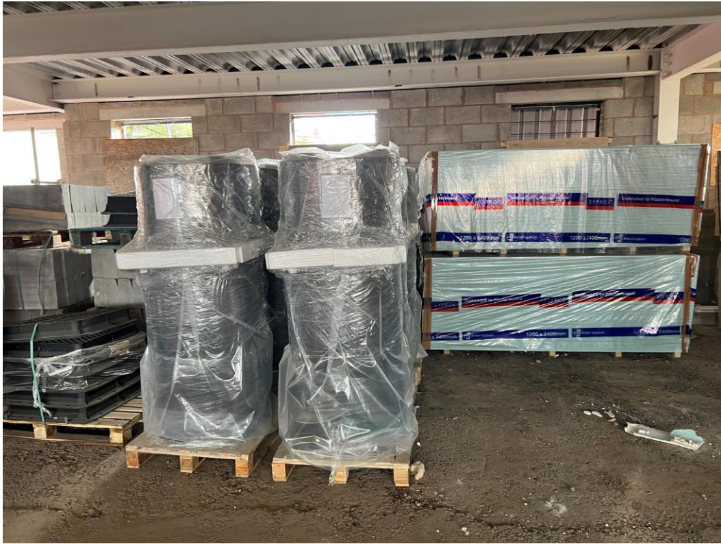
Materials Stored – KERS Units
