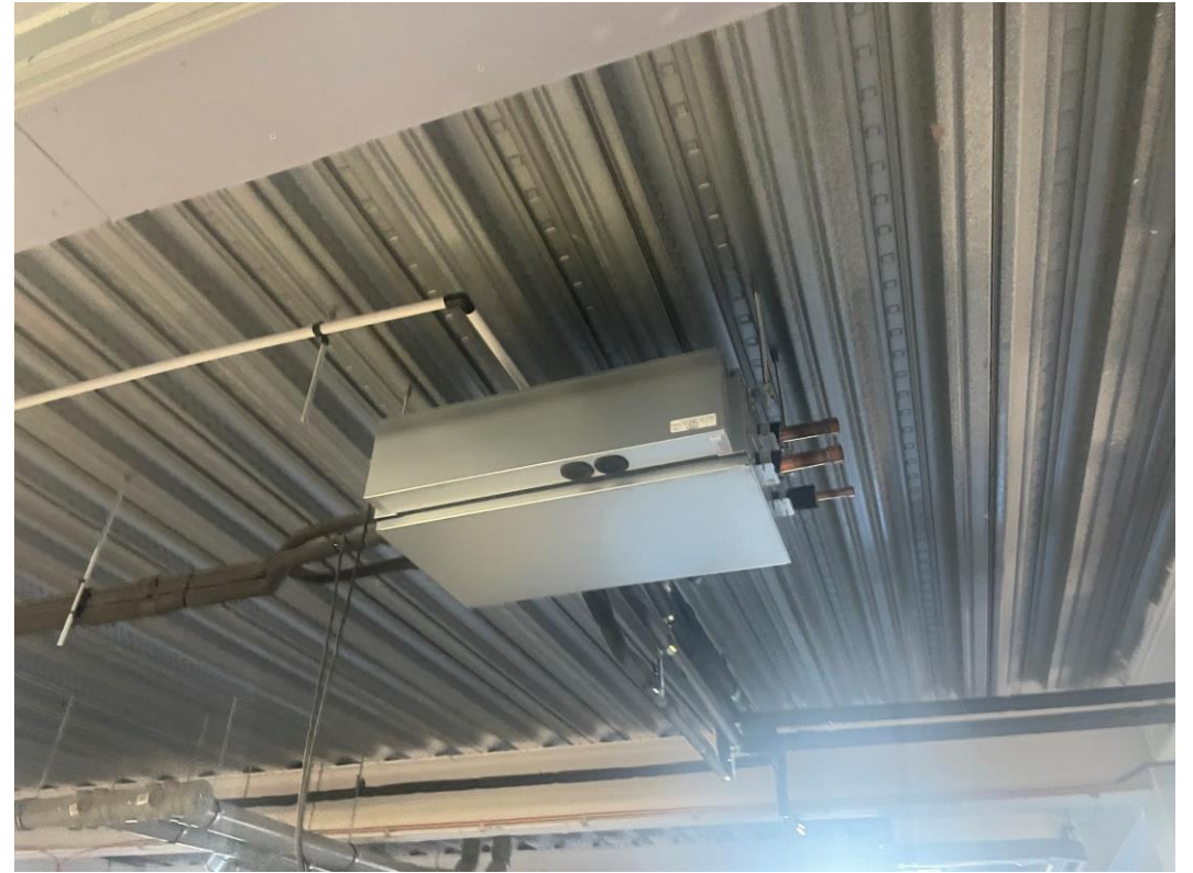
Residential Wing – Air conditioning unit installed
