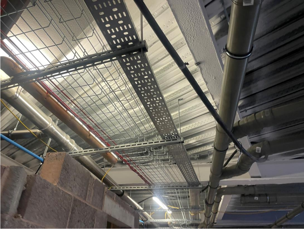
Residential Block – Electrical containment
