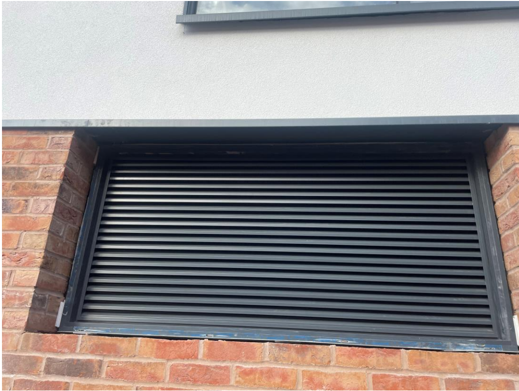
Louvre ventilation grills
