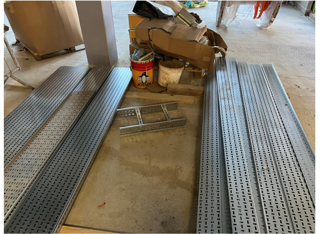
Material Storage – Cable trays
