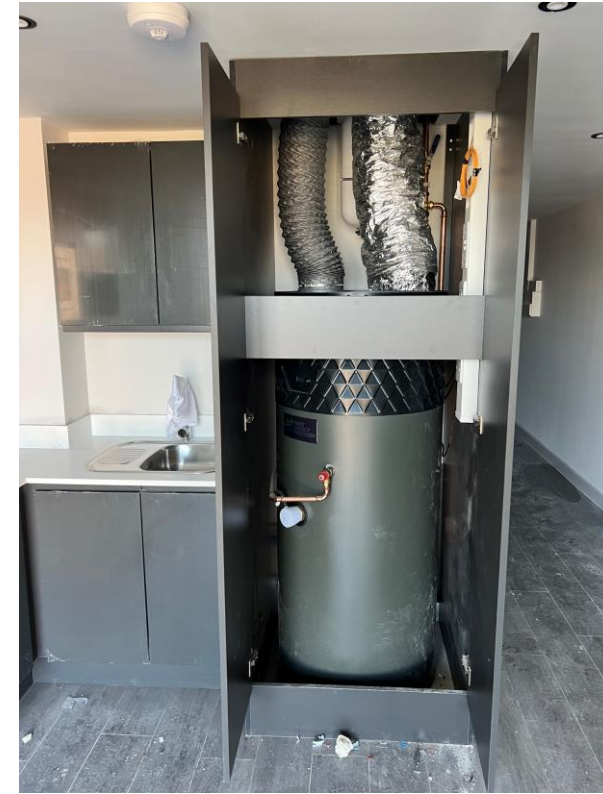
Residential Wing – KERS units installed
