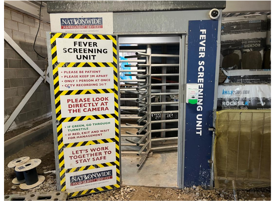
Turnstile being utilised
