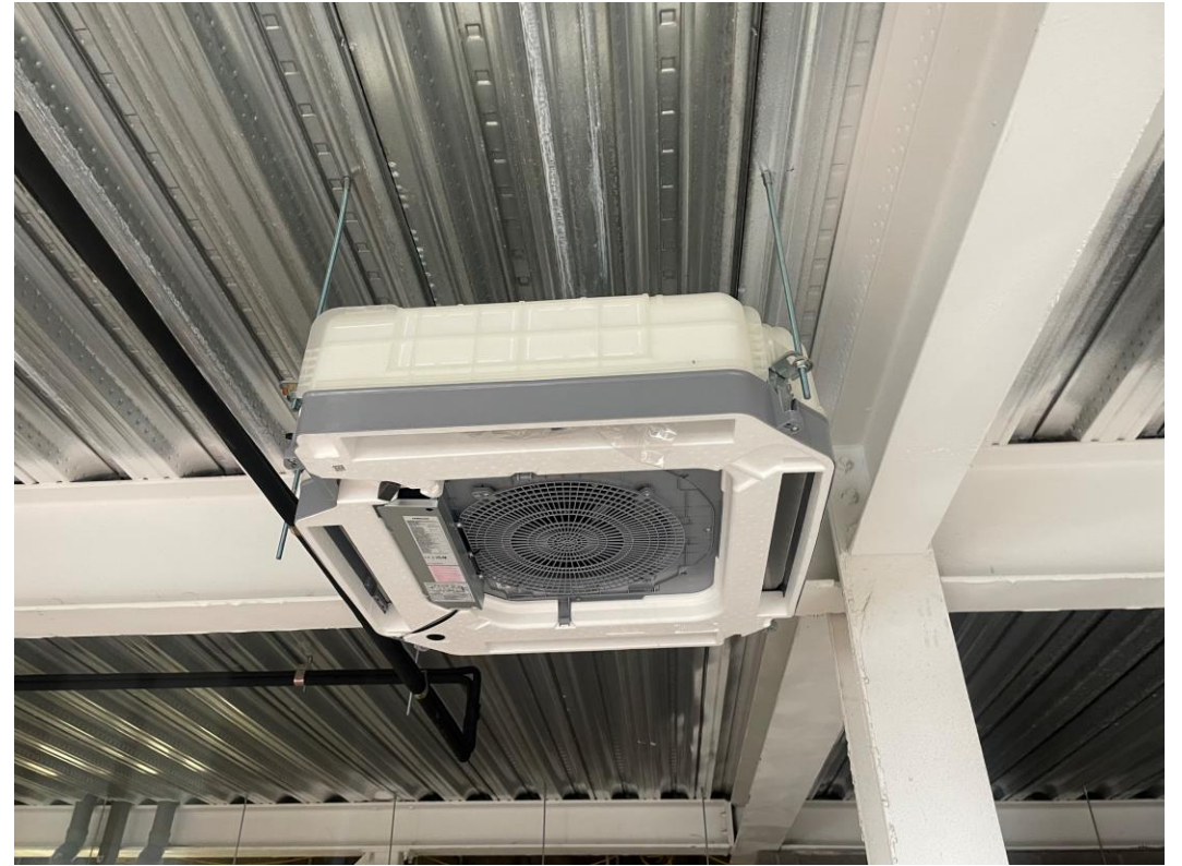
Student Wing – Air conditioning unit installed
