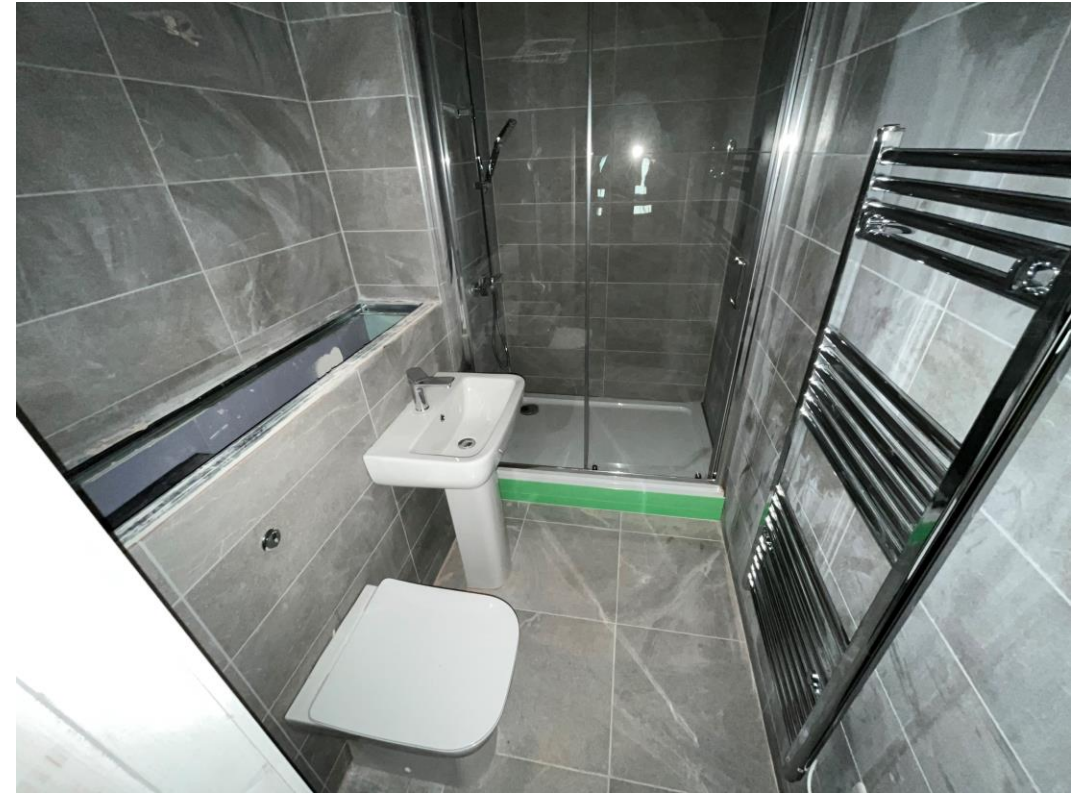
Residential Block – Bathroom sanitary items
