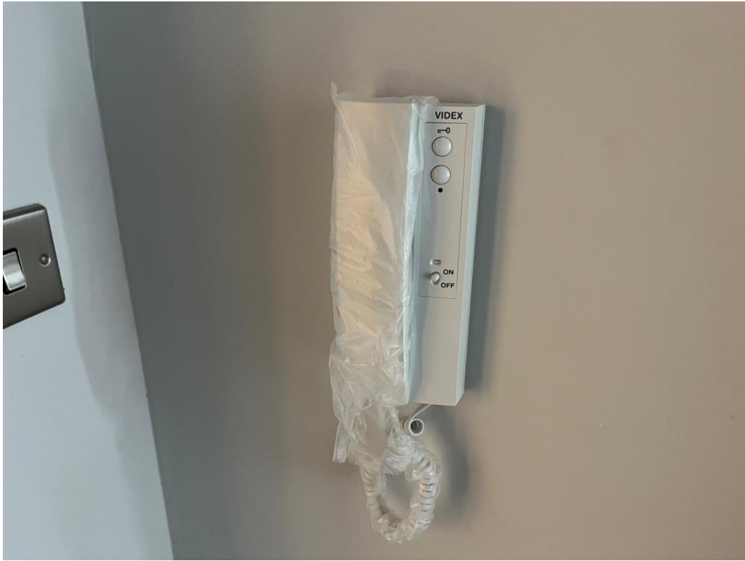
Residential Block – Intercom telephone system
