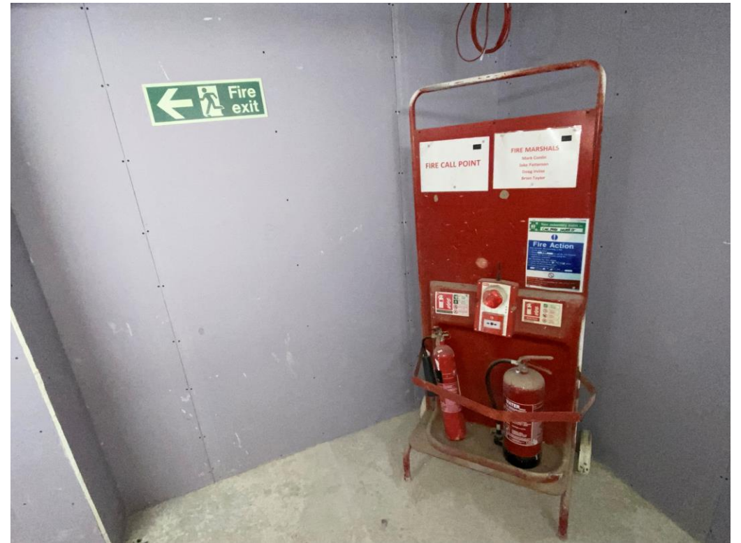
Residential Block – Fire call point
