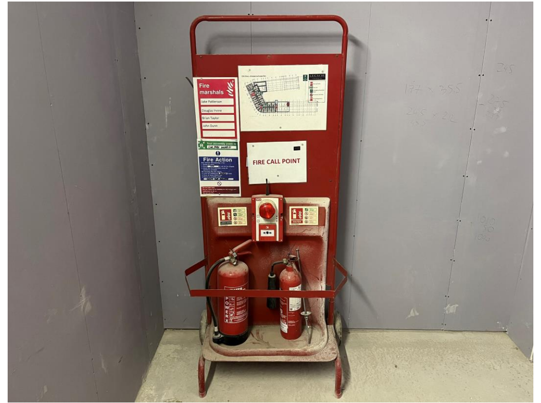
Residential Block – Fire call point
