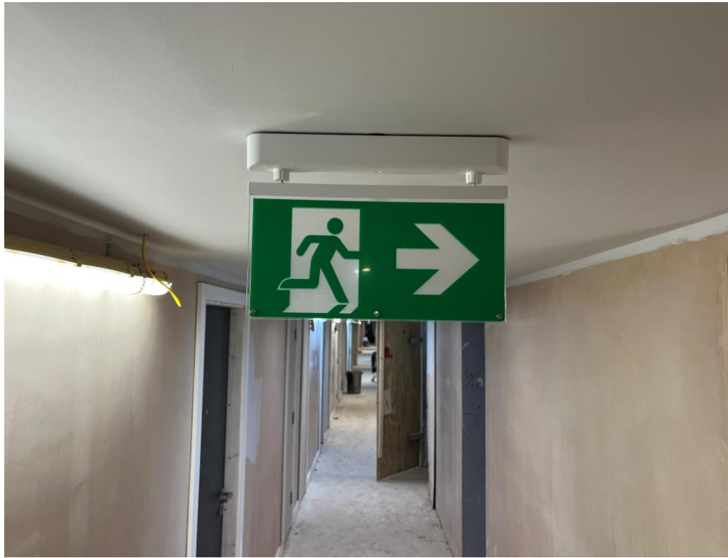
Student Wing – Fire exit signage
