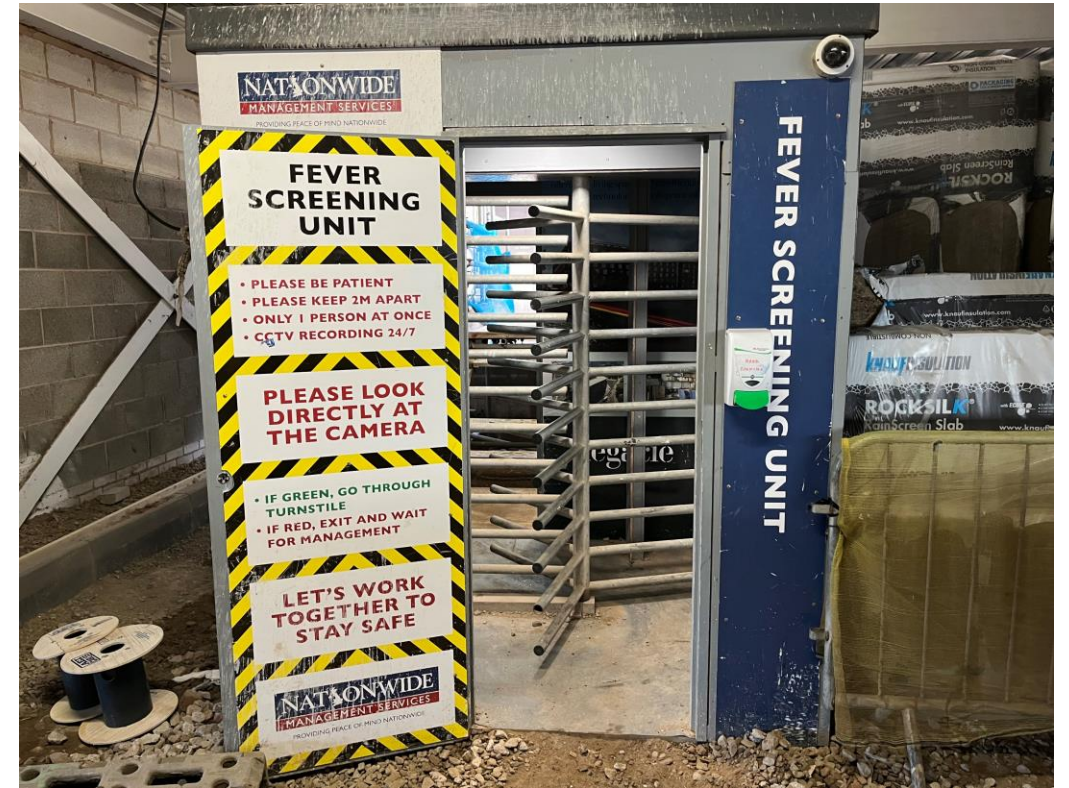
Turnstile being utilised
