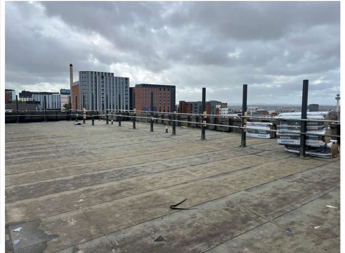
Temporary edge protection installed
