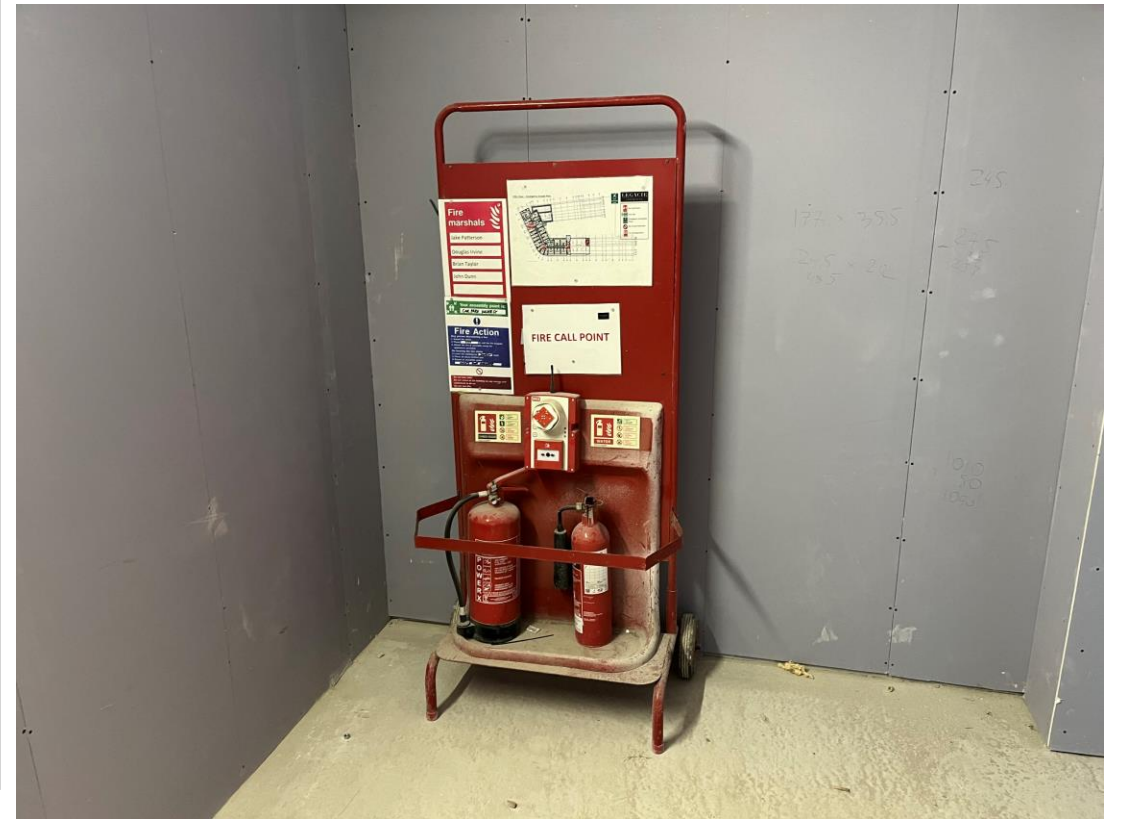
Residential Block – Fire call point
