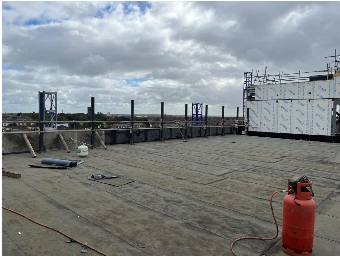
Temporary edge protection installed
