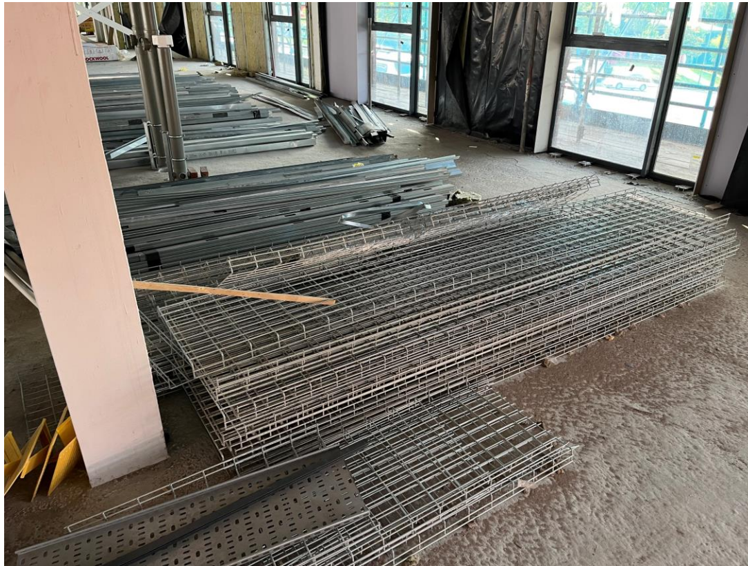
Material storage – Cable trays
