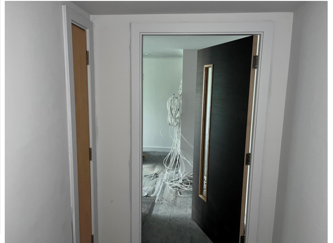
Student Wing – Fire doors
