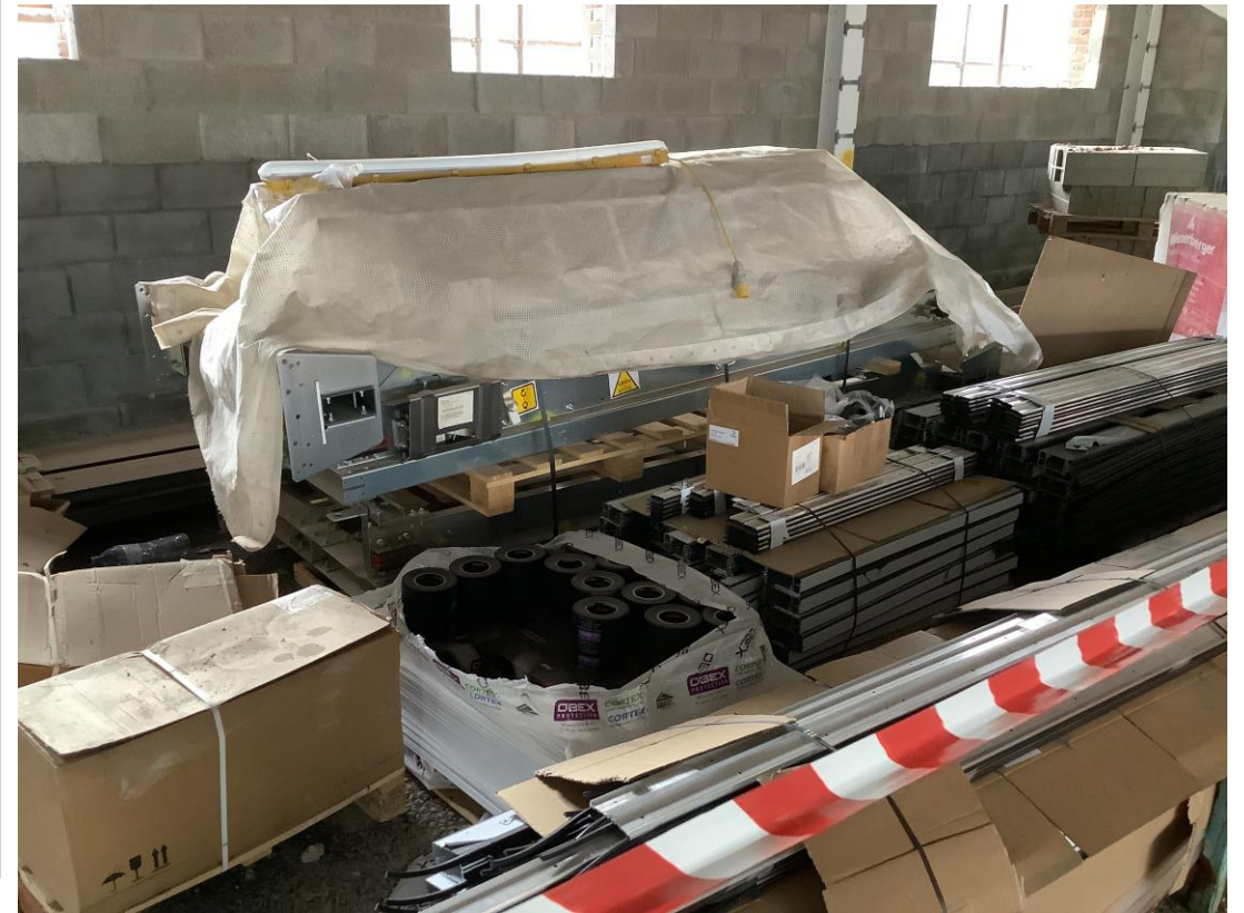
Material storage – Mechanical equipment
