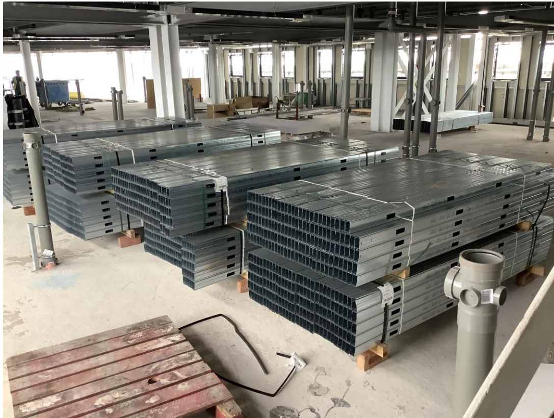
Material storage – Metal trunking
