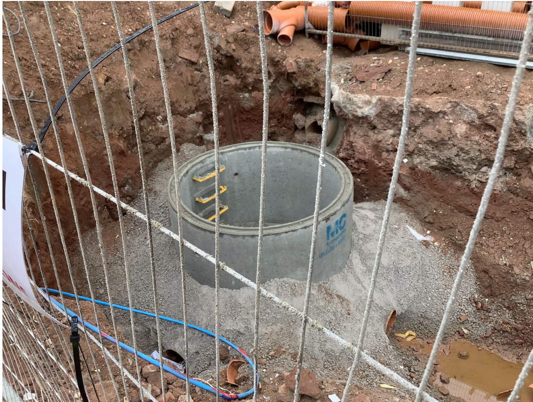
External inspection chamber
