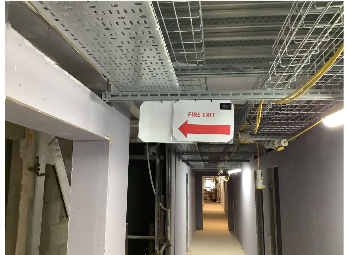
Directional fire exit signage
