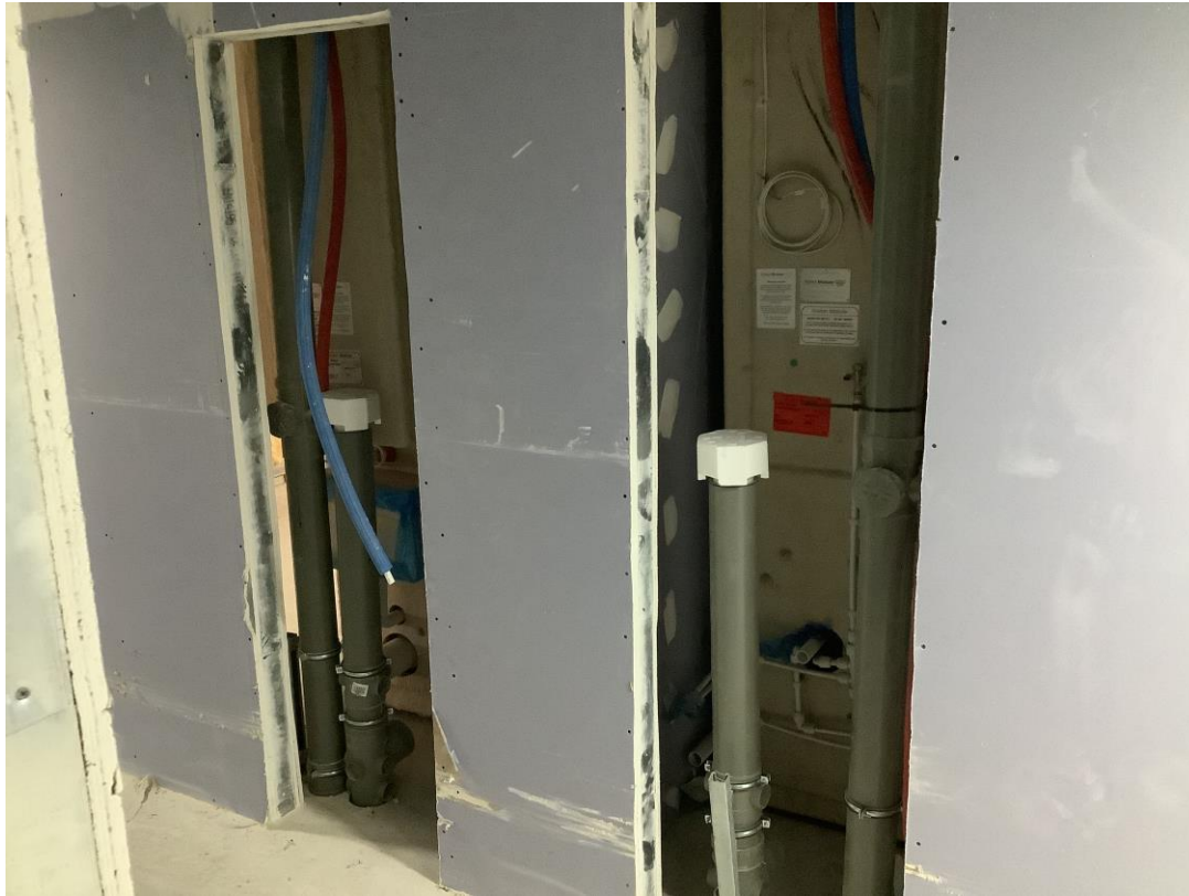
Student wing - Maintenance access hatches
