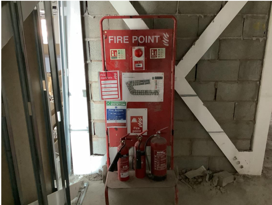
Student wing - Upper floor fire points
