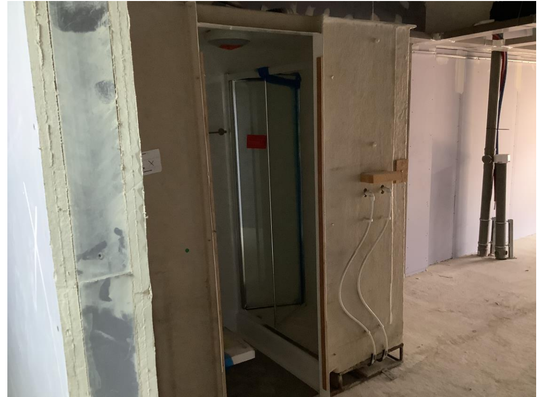
Student wing - Bathroom pod
