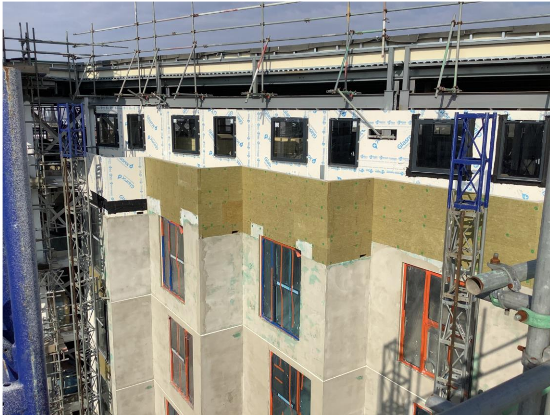
Student wing view of 'Zig zag elevation' - External insulation and render progress
