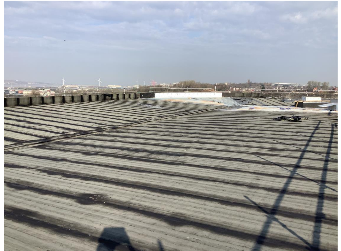
Residential wing - Visqueen layer to flat roofs
