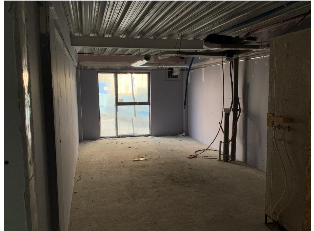
Student wing - Internal metal partition boarded
