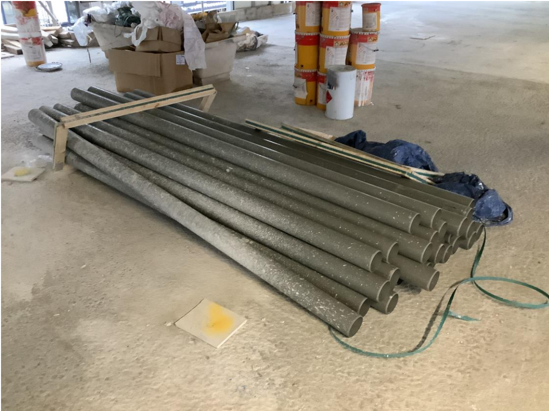
Material storage - Upvc pipes
