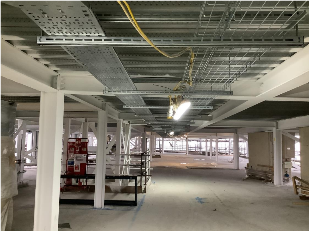
Student wing - Upper floor Electrical containment
