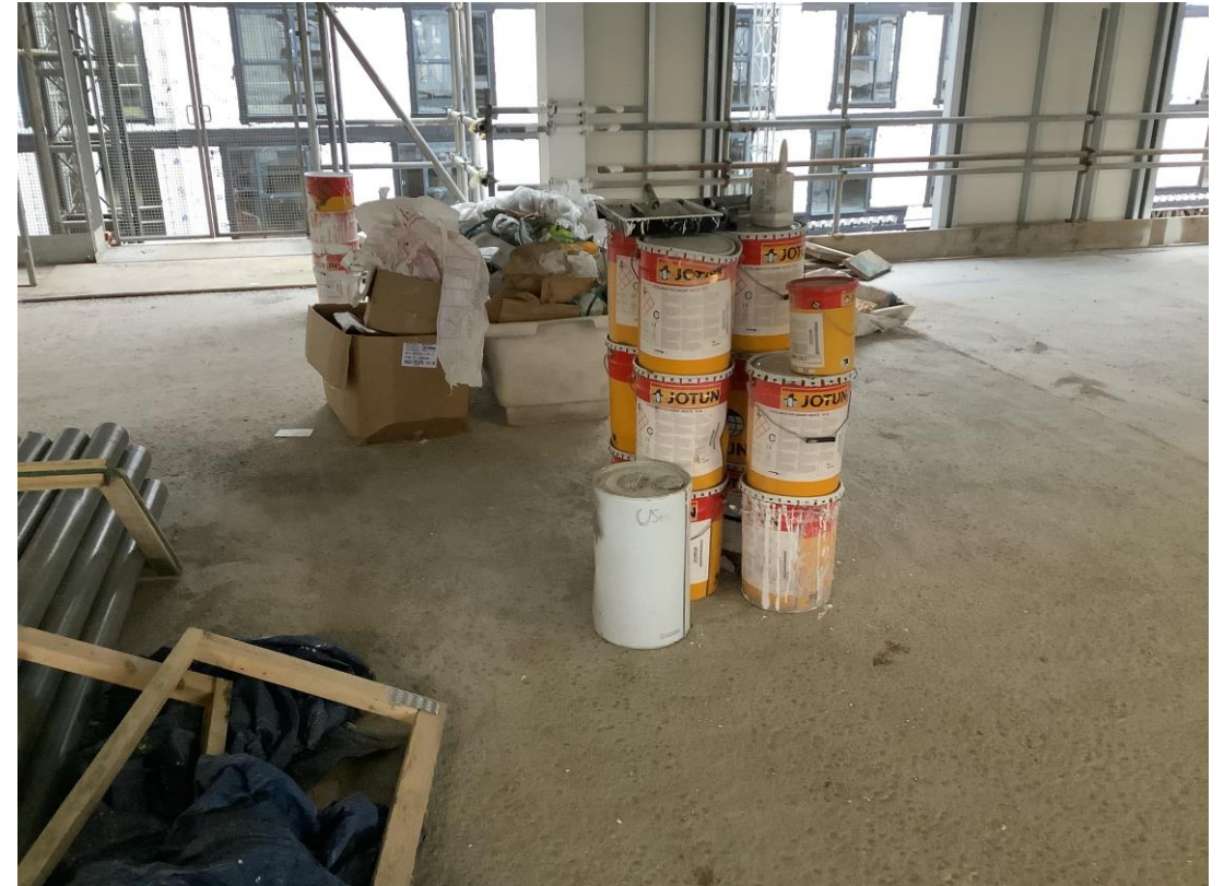
Material storage - Intumescent paint
