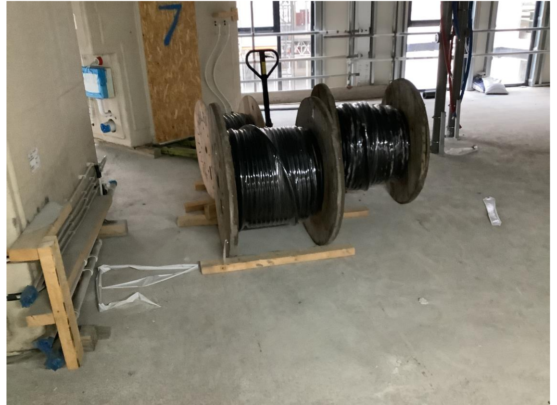
Material storage - Electrical cabling
