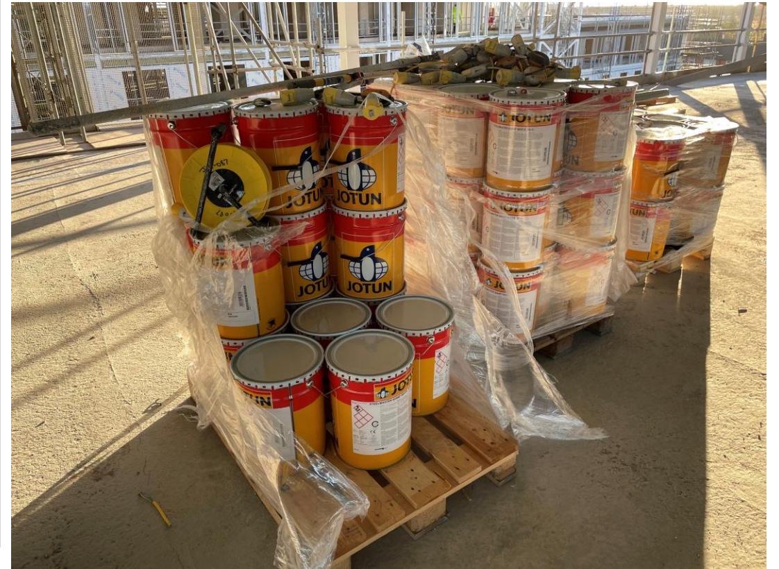
Material storage – Intumescent paint
