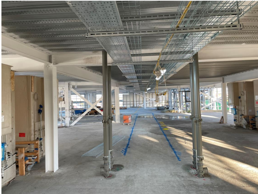
Electrical containment and demarcation to upper floors – Student wing
