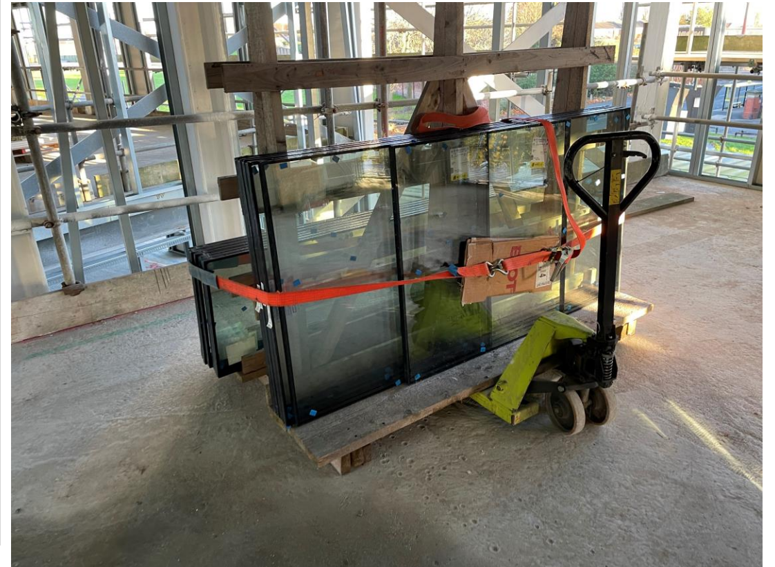
Glazing panels stored on pallet truck in preparation for installation to window units – Student wing
