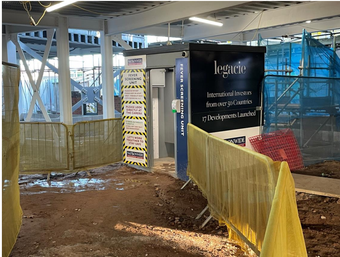
Site barriers and turnstile being utilised
