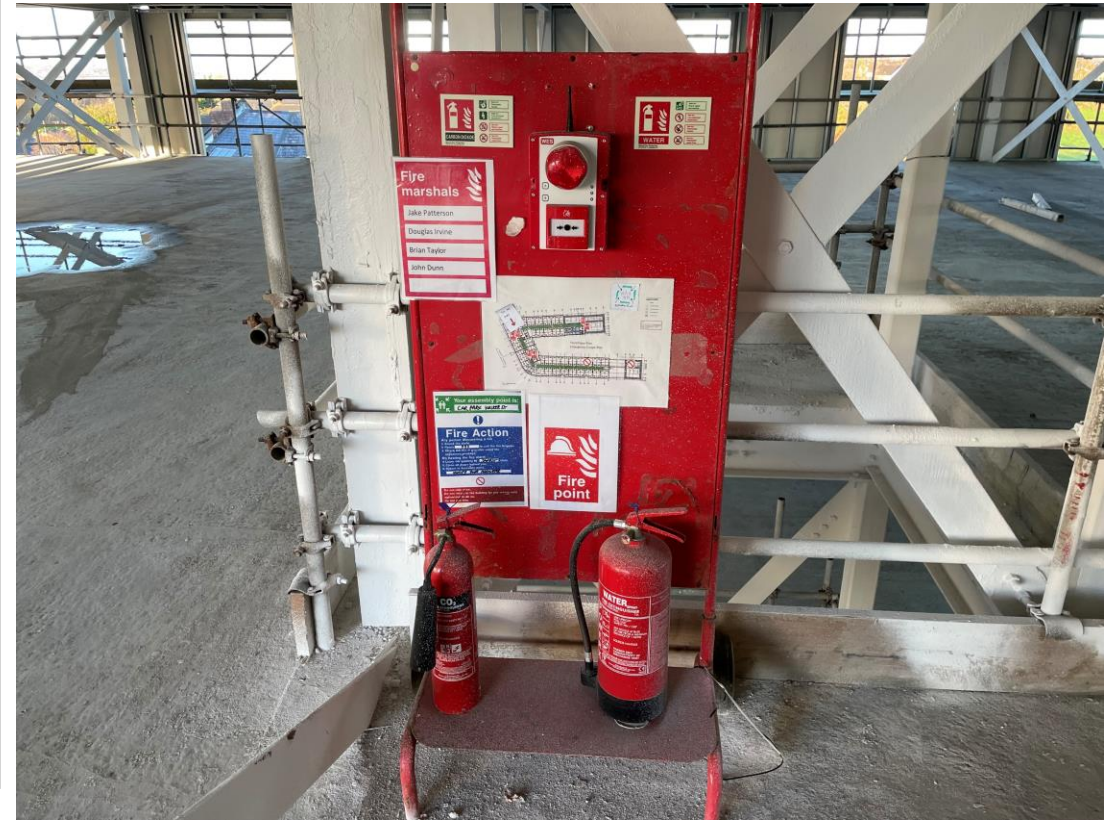
Upper floor fire point
