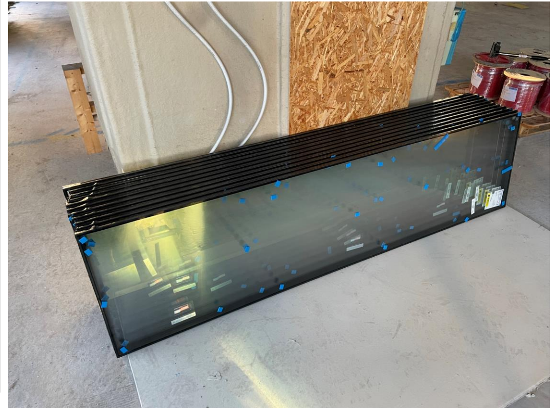
Glazing panels stored in preparation for installation to window units – Student wing
