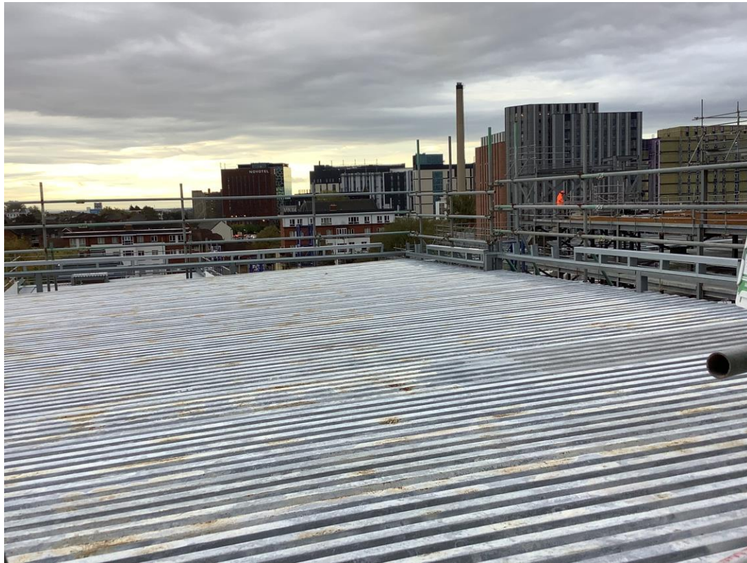
Metal decking structure to upper floors – Upstand to parapet alterations on going
