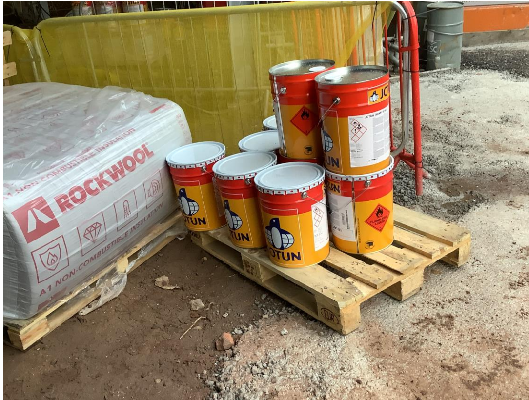
Material Storage – Intumescent Paint
