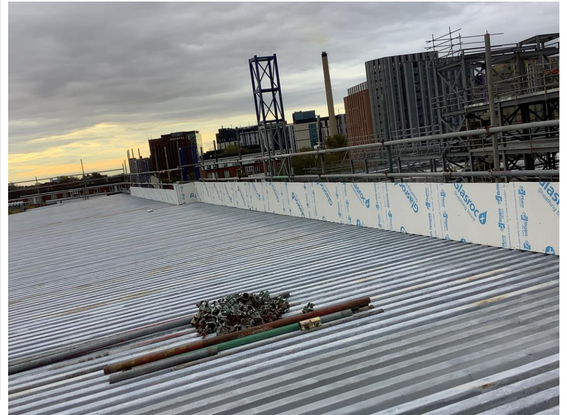
Metal decking structure to upper floors – Upstand to parapet alterations on going
