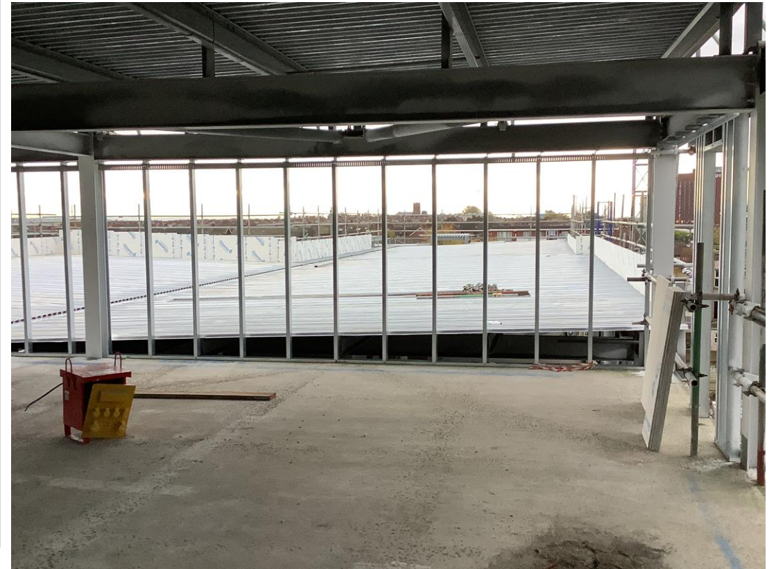
Metal decking structure to upper floors – Upstand to parapet alterations on going
