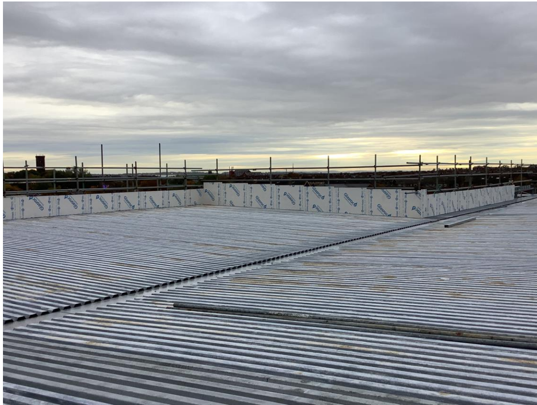
Metal decking structure to upper floors – Upstand to parapet alterations on going
