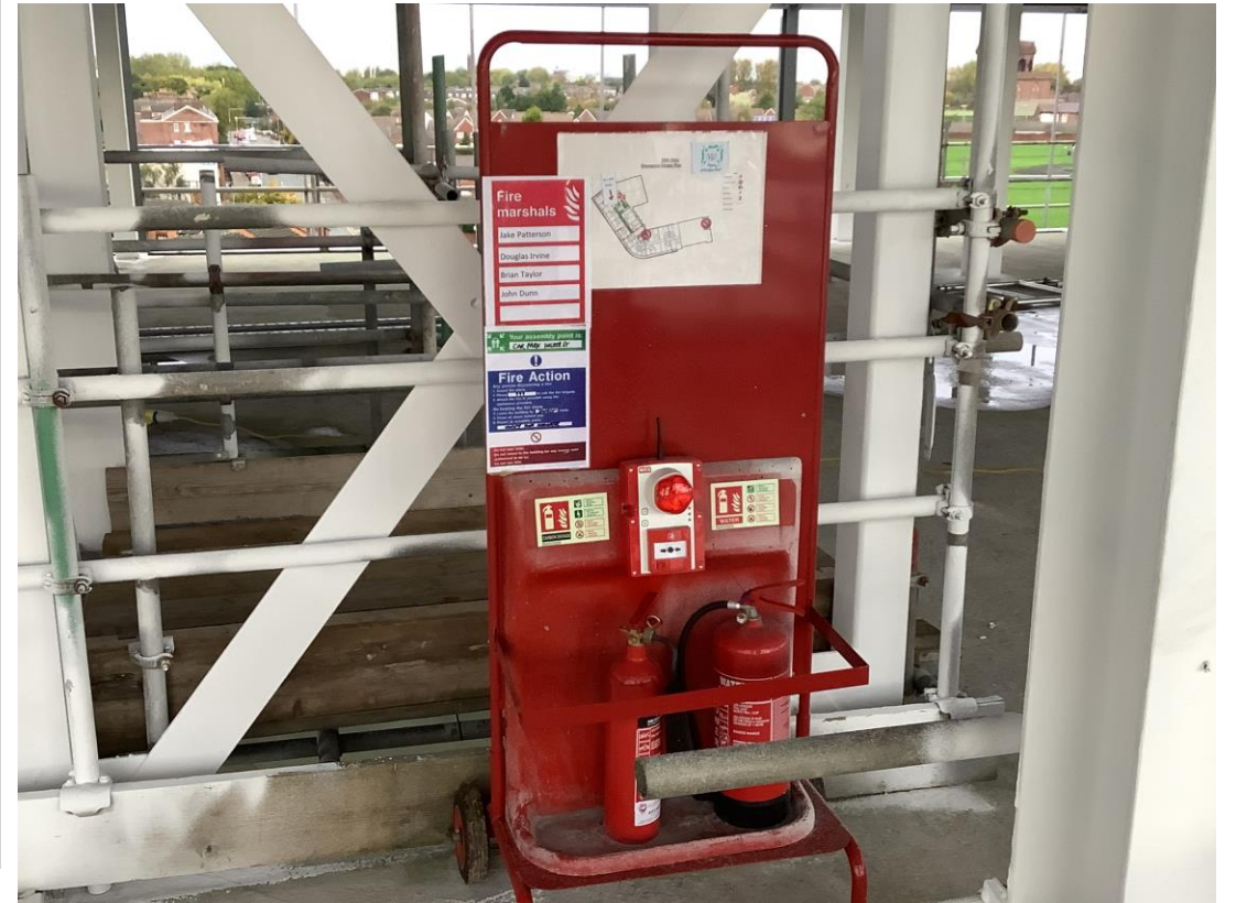
Upper floor fire point
