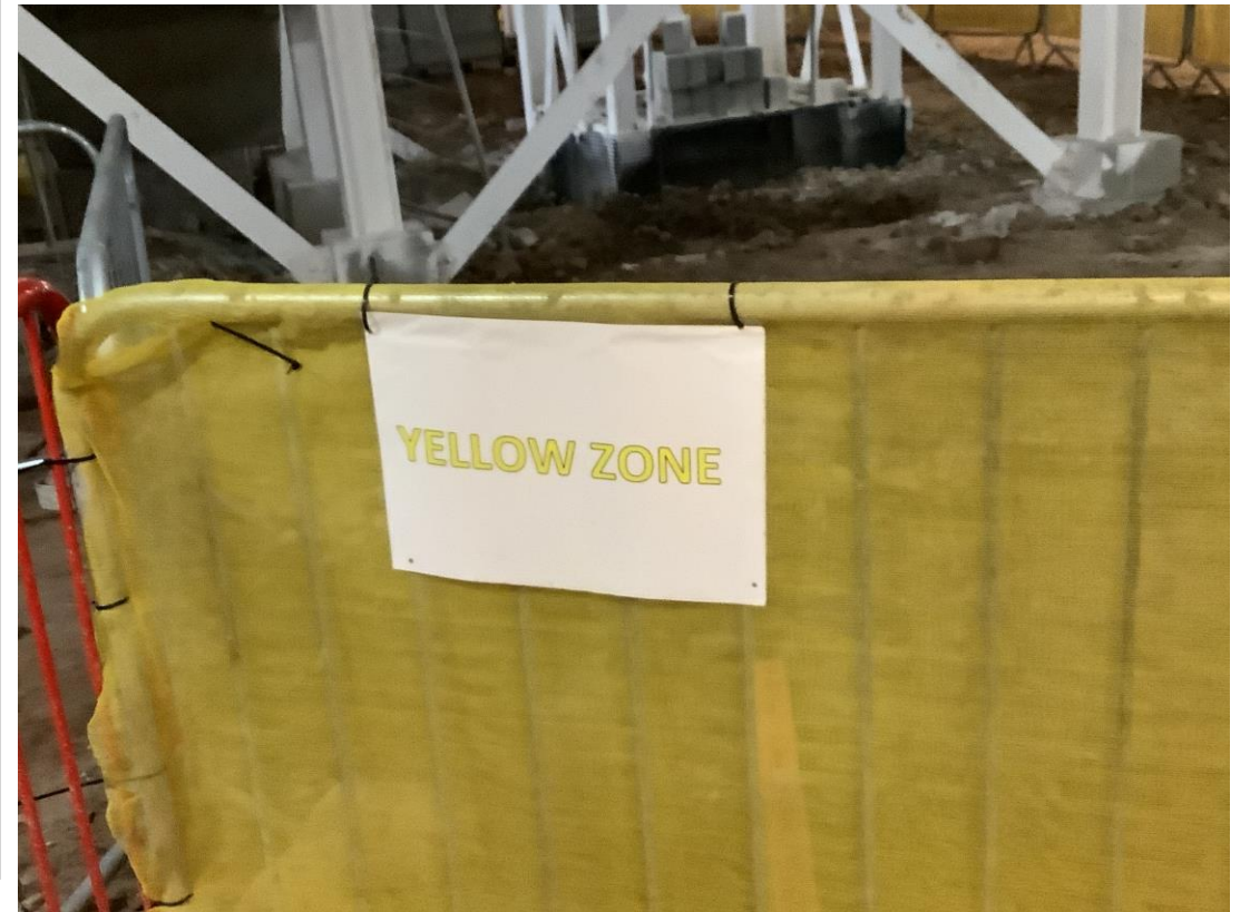
Safe zones installed
