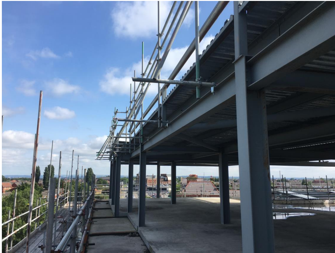
Steel framework structure to upper floors – Steel frame modifications and balcony removal to be complete
