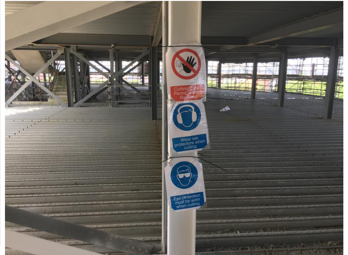
Temporary health and safety signage
