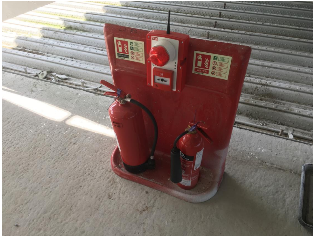
Fire call point adjacent to stair core
