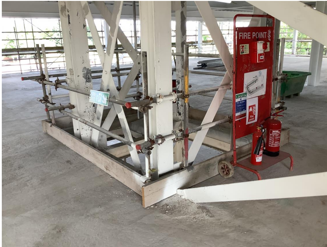
Upper floor fire point
