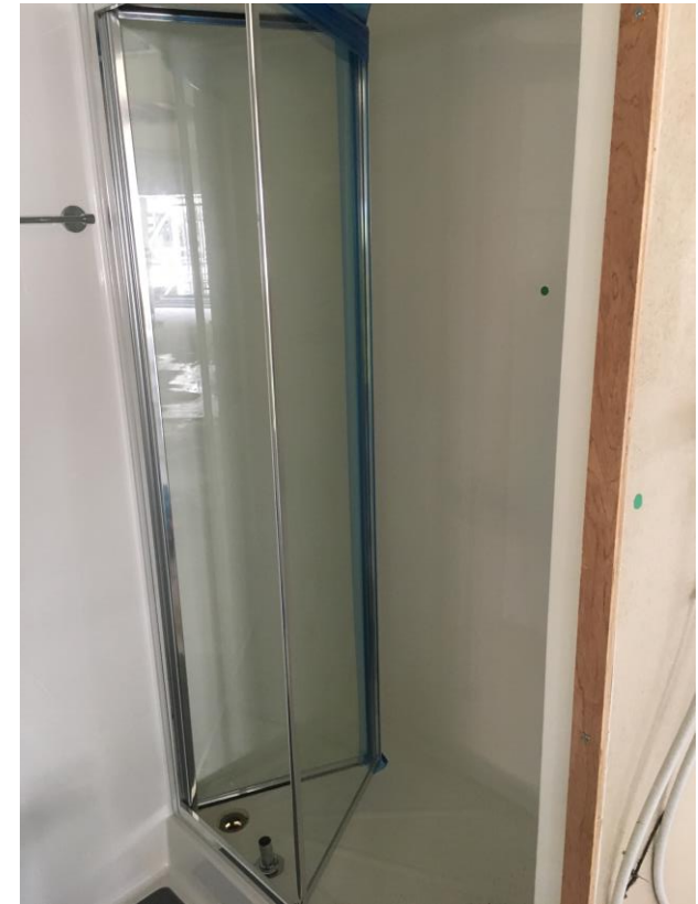
Bathroom pods delivered for installation - Pod testing and itinerary checks currently ongoing
