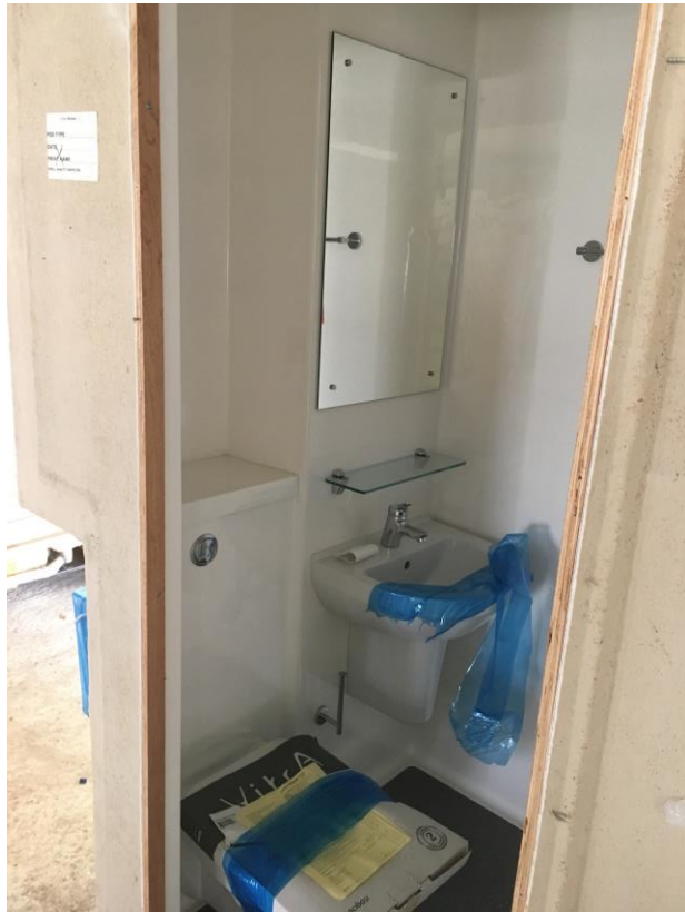
Bathroom pods delivered for installation – Pod testing and itinerary checks currently ongoing
