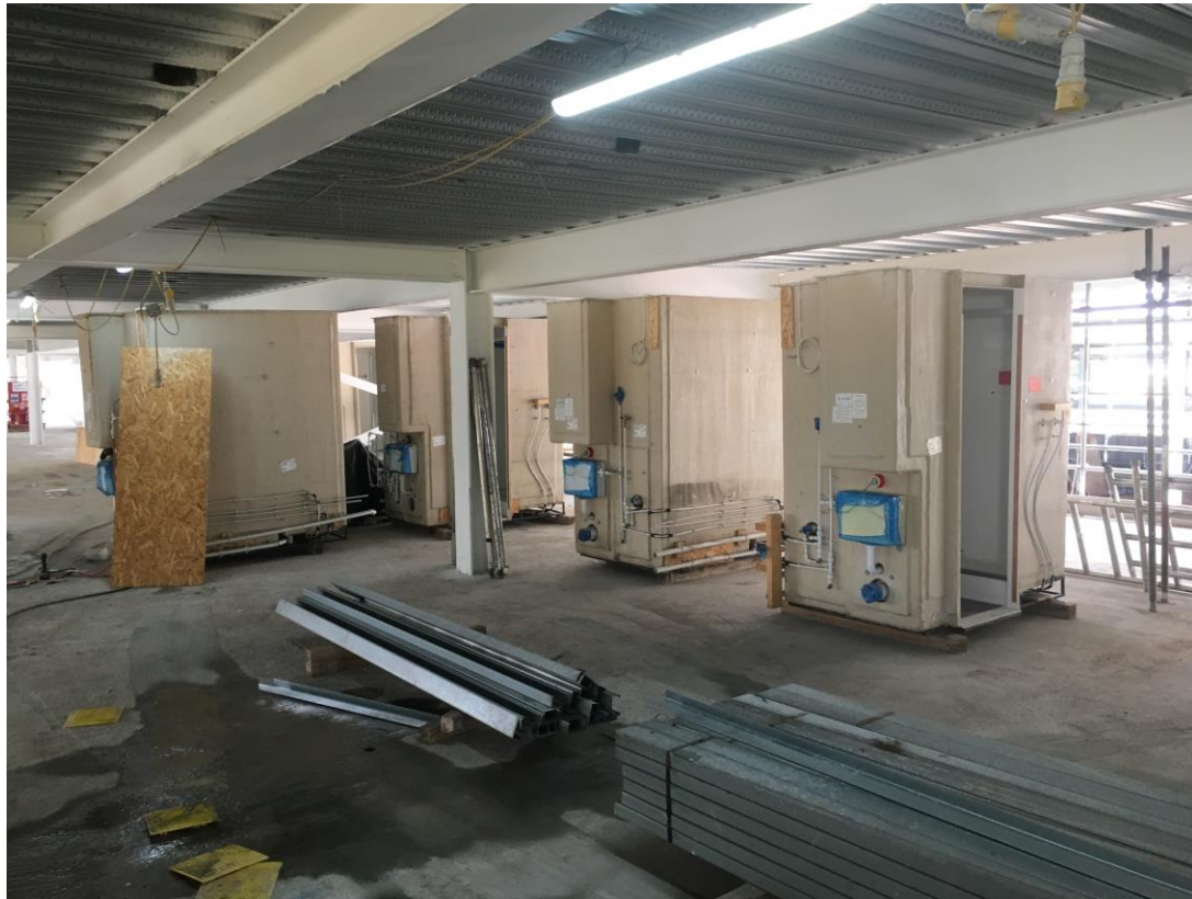
Bathroom pods delivered for installation – Pod testing and itinerary checks currently ongoing
